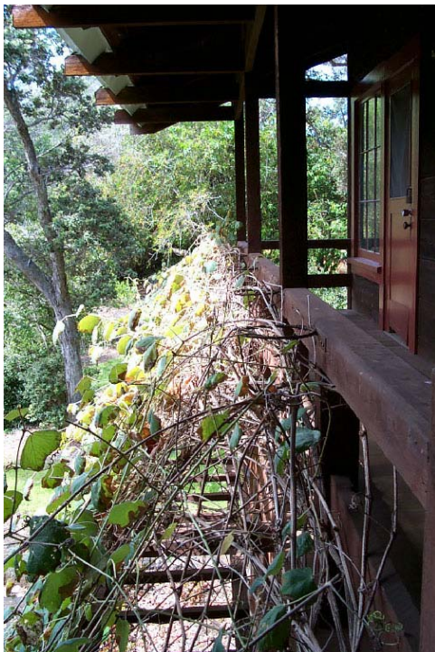
Buildings and Structures # 2: Contemporary photo of the grape trellis located on the south side of the ranch house (PWR, HAVO, CLI files, 2003).
