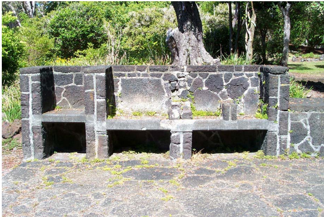
Buildings and Structures # 5: Contemporary photo of the barbecue pits built with lava rocks in a mosaic pattern (PWR, HAVO, CLI files, 2003).
