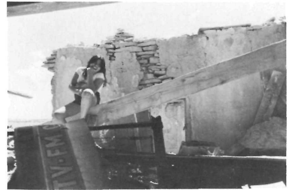
Some of the walls need only to be strengthened and then replastered. Others can be dismantled and the stones reused. Because of New Mexico's dry climate, most of the vigas have been preserved and can be used again for new roofs.
