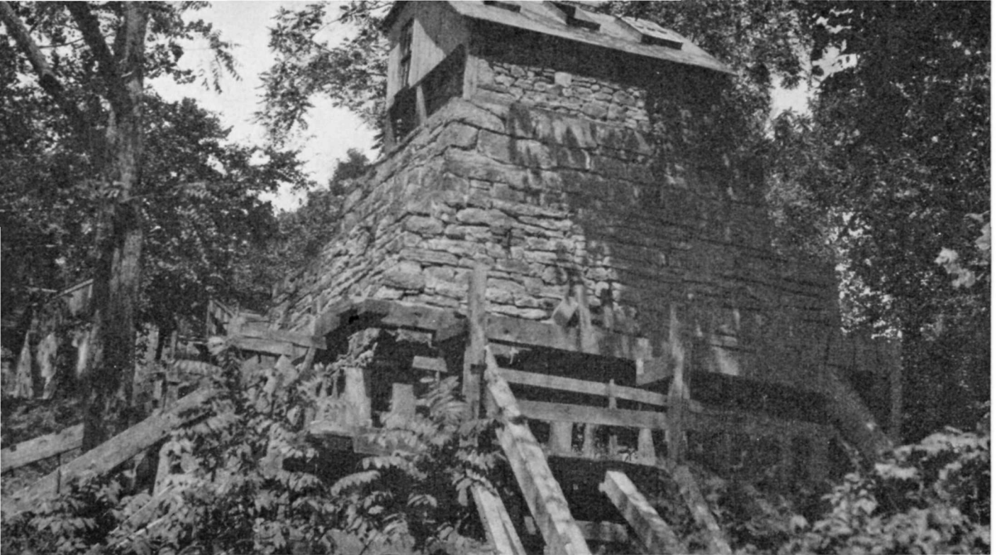
Stabilization of Hopewell Furnace is being accomplished by working from the top down, inside the stack, on small sections at a time. This involves removing all stonework except the outermost layer, which is not touched except to repair breaks; and then replacing the inside stonework with concrete and steel reinforcing in place of the old lime mortar
