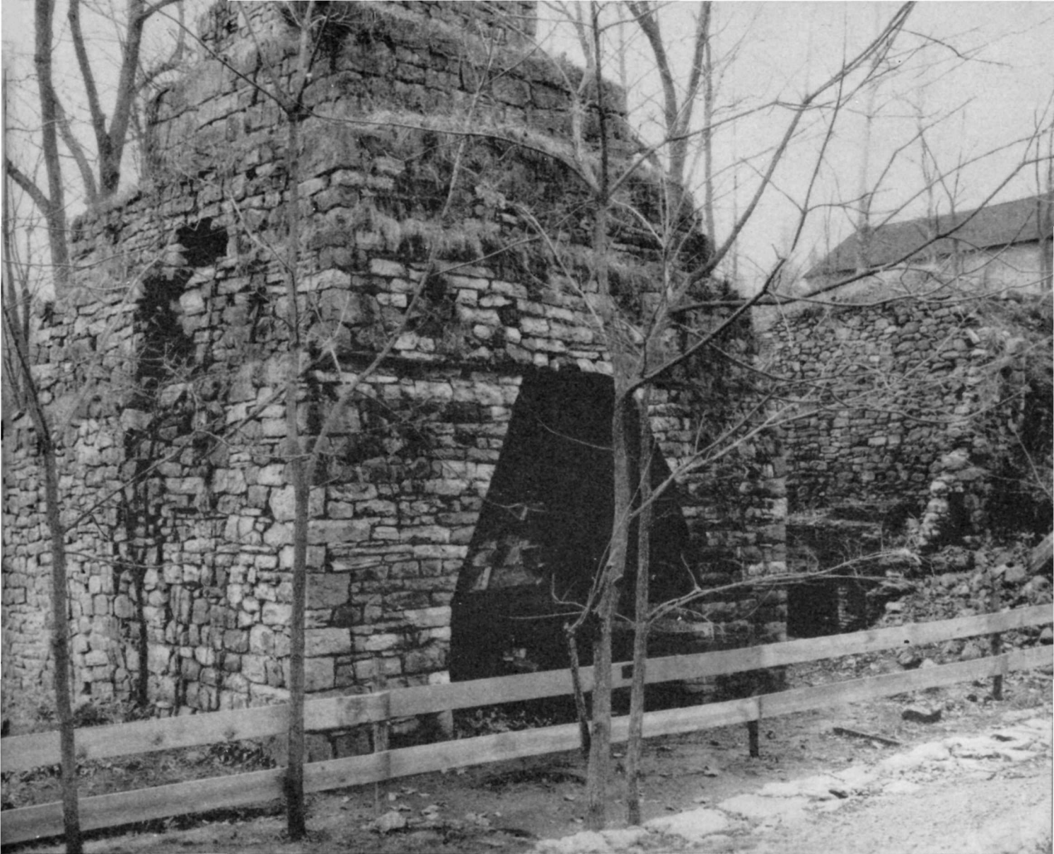
Hopewell Furnace before stabilization. This picture shows one of several large fissures in the furnace stack resulting from frost, vegetative growth, and other elemental forces operating since 1883, when the old stack closed down for good after more than a century of activity
