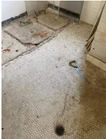
XAI.82 – Shower 220. Damaged tile flooring.
