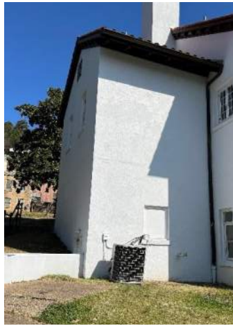
XP.5 Abandoned Gas Service
