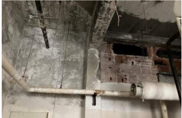
XAI.16 – Mechanical 107. Damaged plaster and holes cut into clay tile walls.
