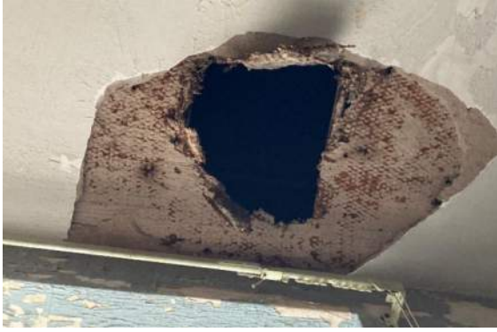
XAI.19 – Office 109. Damaged plaster at ceiling.
