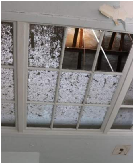
XAI.63 – Hallway 209. Damaged laylight.
