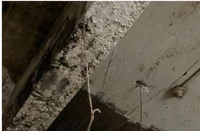
XAI.17 – Mechanical 107. Deterioration at concrete beam.
