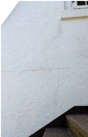
XAE.11 – Cracking at exterior wall paint and stucco.
