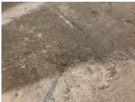
XAI.28 – Mechanical 114. Pitted concrete floor.
