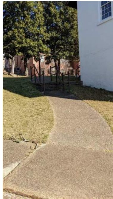
XC.6 – Exterior at West. Damaged sidewalk, railing at stair.
