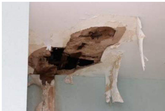
XAI.69 – Treatment Room 211. Damaged ceiling plaster.
