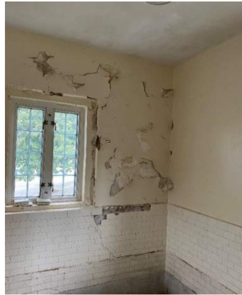
XAI.79 – Men's Bath 218. Damaged plaster wall and tile.
