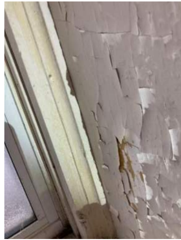
XAI.23 – Toilet 111. Damaged plaster and paint at window jamb.
