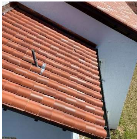
XAE.8– Damaged clay tile.
