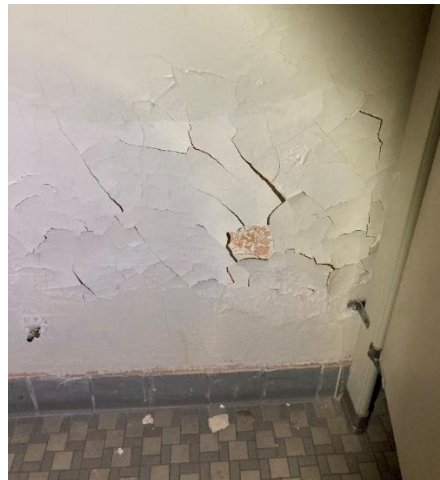
XAI.11 – Toilet 105. Cracked wall plaster and paint.
