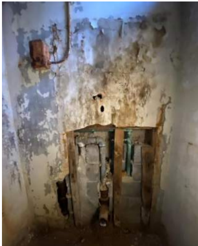
XAI.39 – Mechanical 119. Damaged plaster wall.
