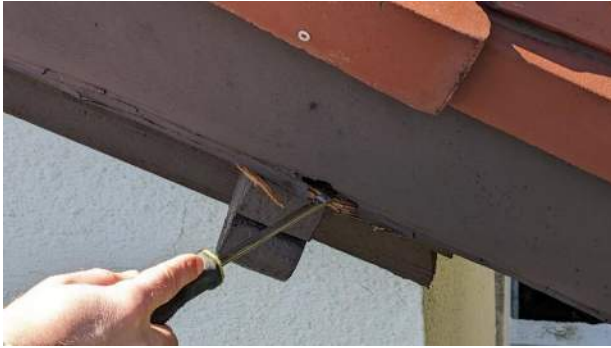
XAE.10 – Damaged wood at soffit and eave.
