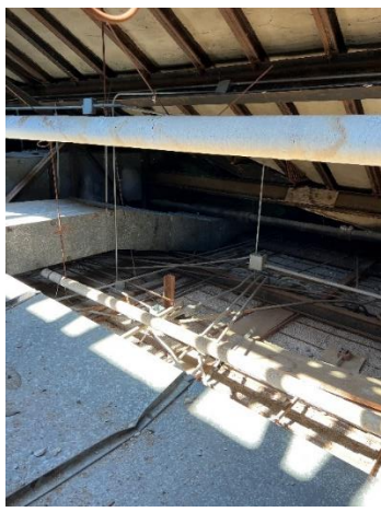
XE.17 Missing Knock Outs
