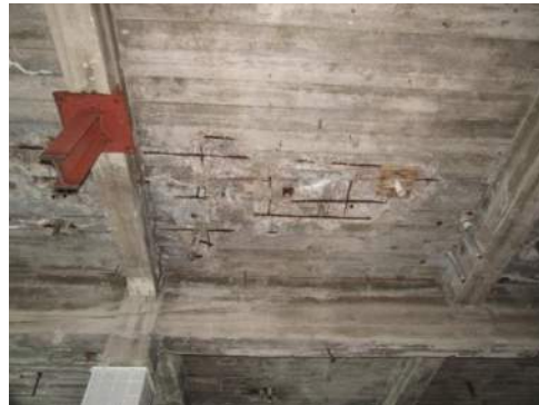
S.2 – Typical overhead slab repair area due to corrosion of reinforcing steel.
