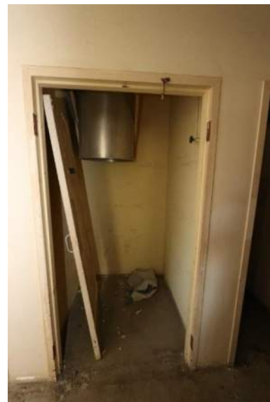
XAI.24 – Laundry 112. Damaged door frame and removed door.
