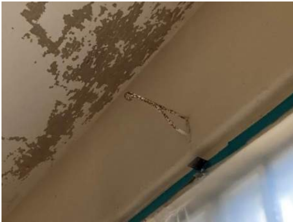
XAI.77 – Room 217. Damaged plaster at ceiling and wall hook above window.
