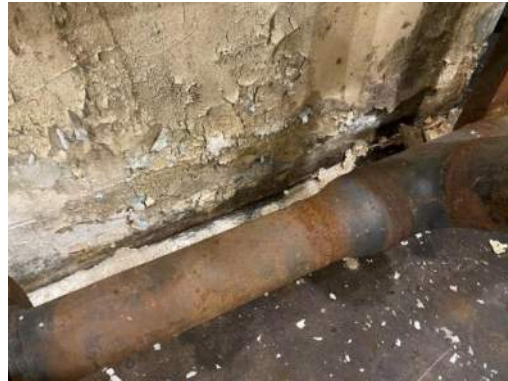
XAI.29 – Mechanical 115. Deteriorated plaster wall.
