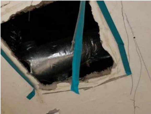
XAI.76 – Room 217. Damaged plaster at ceiling.
