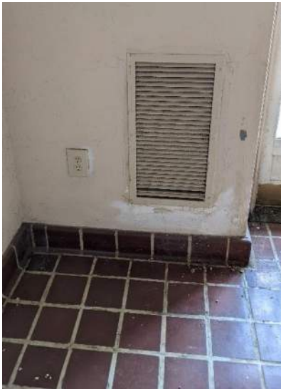
XAI.45 – Lobby 200. Damaged plaster wall and dirty louver and quarry tile and base.
