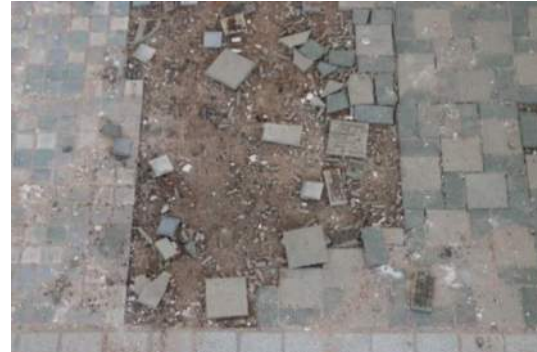
XAI.68 – Treatment Room 211. Damaged floor tile.
