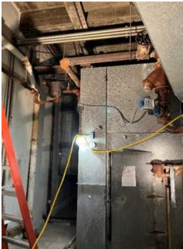
XM.5 Existing Air Handling Unit
