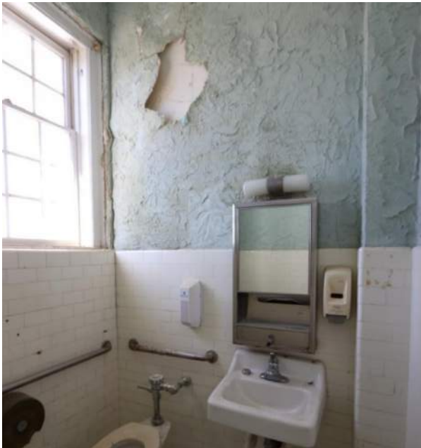
XAI.72 – Toilet 214. Damaged plaster, north wall.
