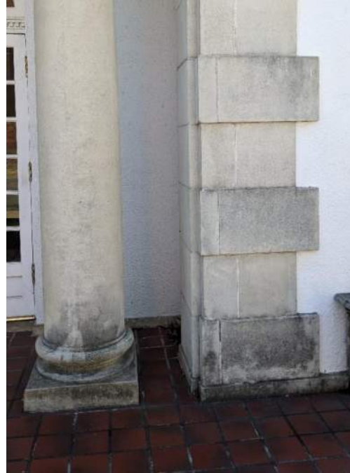
XAE.12 – Atmospheric staining, open joints, and cracking at cast stone column and quoin.
