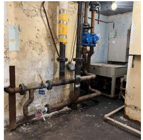
XP.8 Thermal Water Service & Piping
