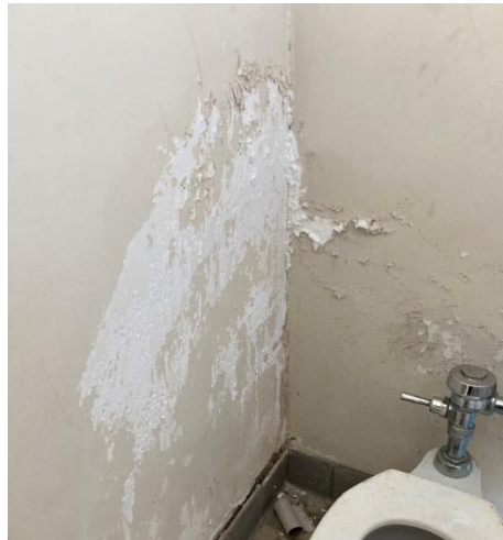
XAI.10 – Toilet 104. Damaged wall plaster.
