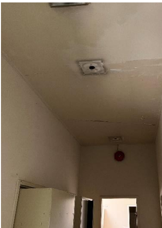
XE.15 Missing Light Fixtures
