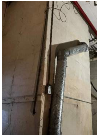
XP.6 Existing Gas Piping
