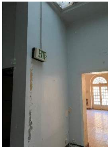
XE.9 Exit Sign
