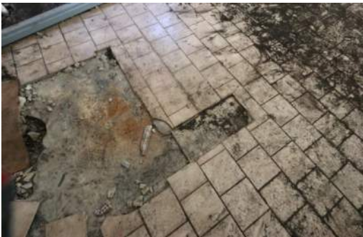
XAI.34 – Pool Room 117. Damaged floor tiles
