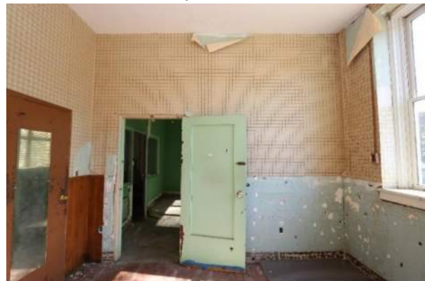
XAI.5 – Office 102. Damaged plaster and peeling wallpaper.
