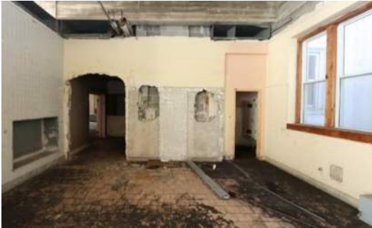
XAI.33 – Pool Room 117. Damaged flooring and walls, looking west.
