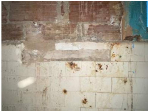
XAI.52 – Pool Room 203. Damaged tiles.
