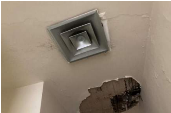
XAI.21 – Toilet 110. Damaged plaster at the ceiling
