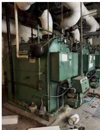
XM.2 Existing Steam Boilers
