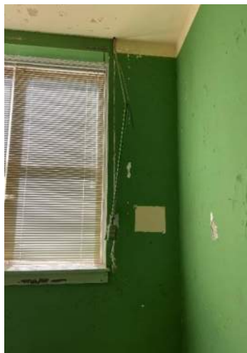
XE.24 Damaged Conduit System
