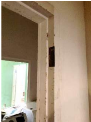
XAI.26 – Room 113. Deteriorated metal door frame.
