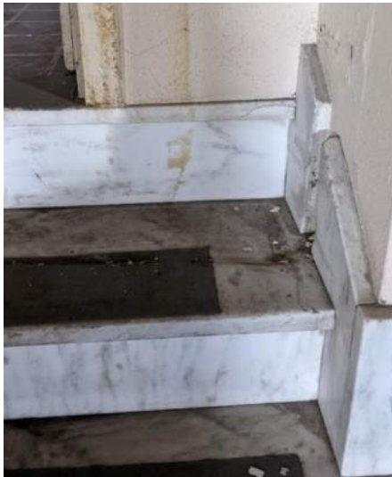
XAI.2 – Stair 100. Damaged marble stair and trim.
