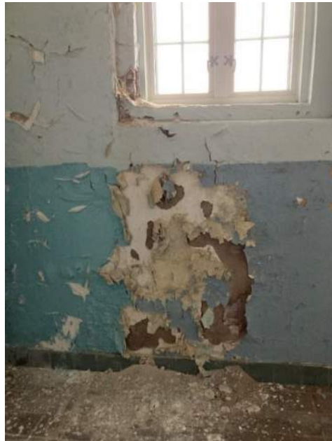
XAI.73 – Room 216. Damaged plaster, south wall.
