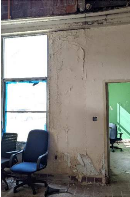
XAI.1 – Lobby 100. Damaged plaster and trim.
