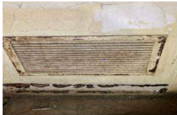
XAI.18 – Office 108. Wall grill and missing wall base.
