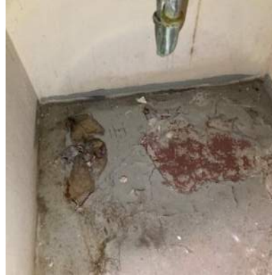
XAI.22 – Toilet 110. Damaged paint at flooring
