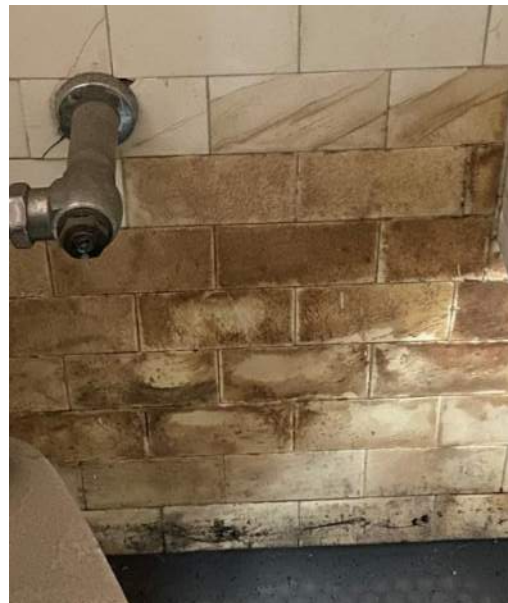
XAI.31 – Toilet 116. Damaged tiles.
