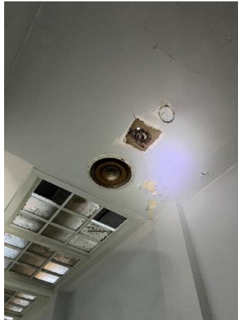
XE.16 Missing Light Fixtures
