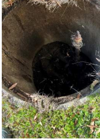
XP.4 Pool Drain Exterior Gate Valve
