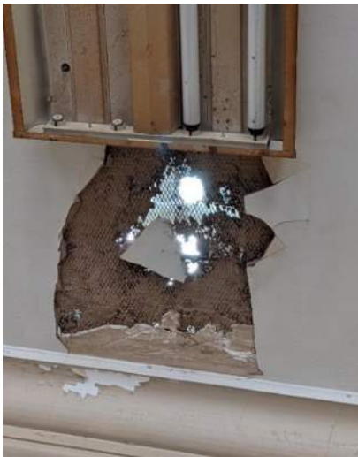
XAI.46 – Lobby 200. Damaged plaster and lighting in ceiling.
