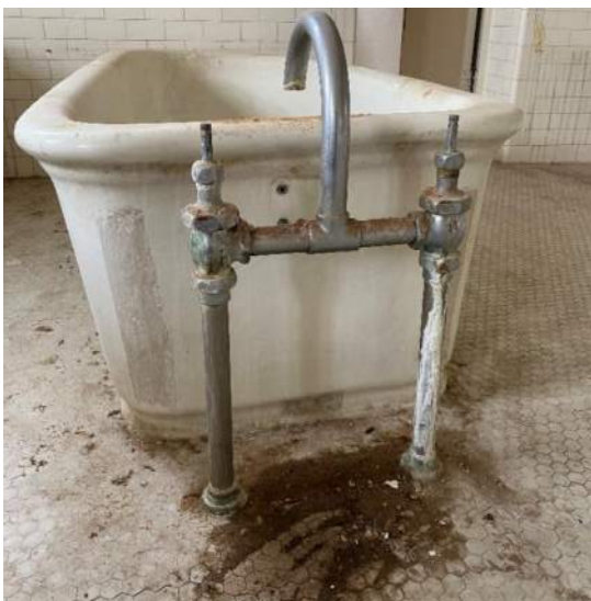
XAI.78 – Men's Bath 218. Damaged flooring, plumbing, and wall tiles.
