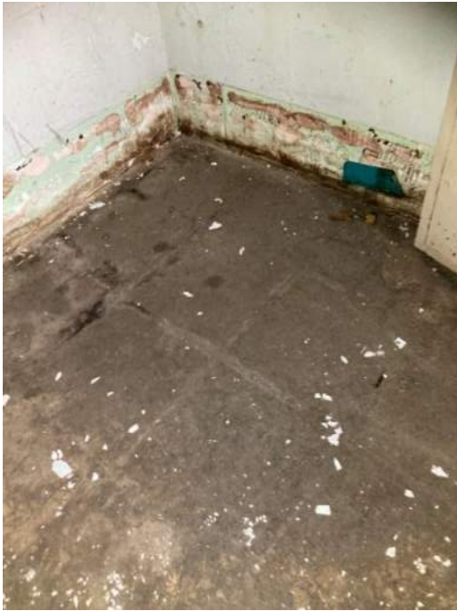
XAI.87 – Toilet 223. Damaged plaster at base of wall.
