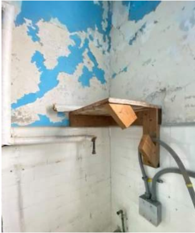
XAI.57 – Toilet 205. Damaged plaster and abandoned pipes.
