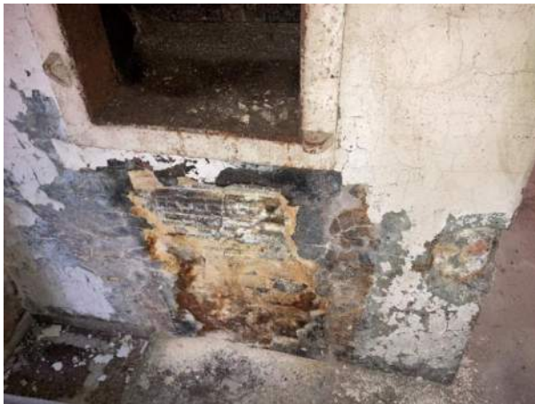
XAI.13 – Mechanical 106. Damaged wall plaster.
