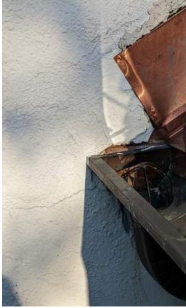
XAE.9 – Damaged stucco wall, around gutter.
