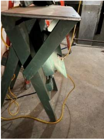
XE.31 Temporary Electrical Equipment
