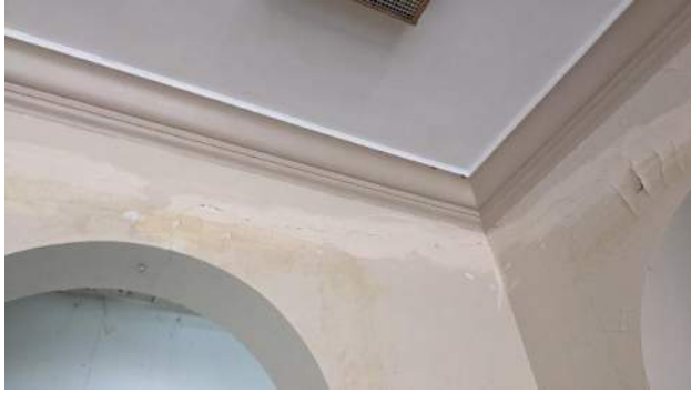
XAI.44 – Lobby 200. Cracked wall plaster.
