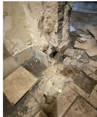
XAI.43 – Hallway East 121. Damaged Floor
