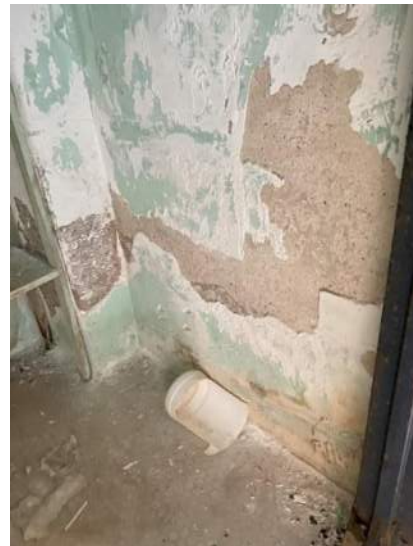
XAI.55 – Closet 204. Damaged plaster.
