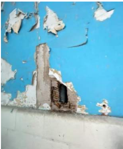
XAI.59 – Toilet 206. Damaged wall plaster.
