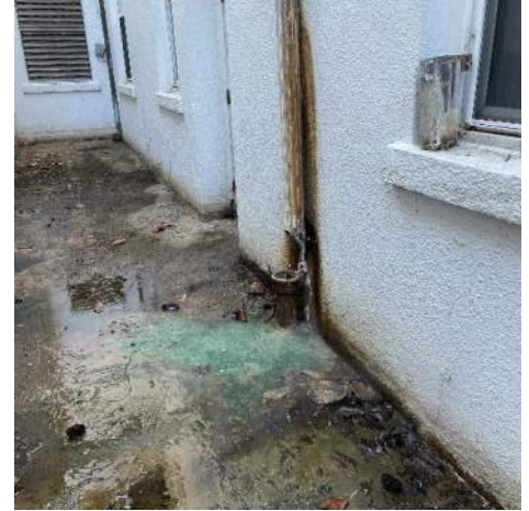
XP.7 Missing Section of Downspout Leader
