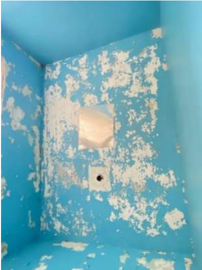
XAI.58 – Toilet 206. Damaged ceiling plaster.
