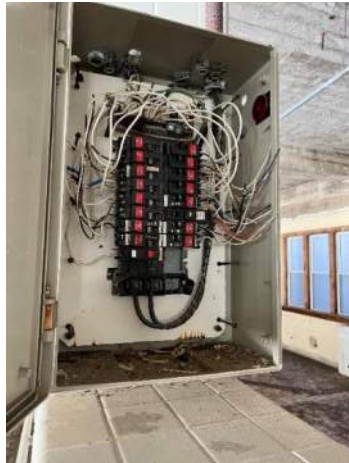
XE.32 Incomplete Wiring
