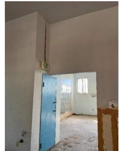
XE.30 Existing Exit Sign
