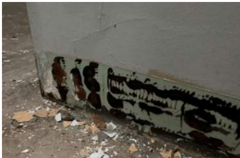
XAI.64 – Hallway 209. Missing wall base.
