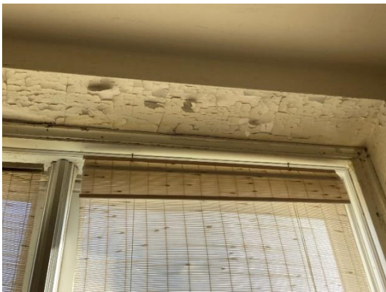
XAI.8 – Office 103. Damaged at window header.
