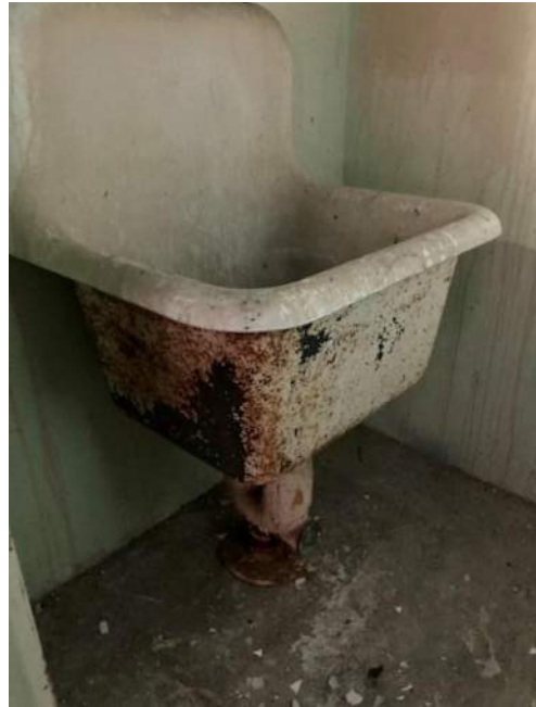
XAI.89 – Janitorial Closet 224. Damaged sink.
