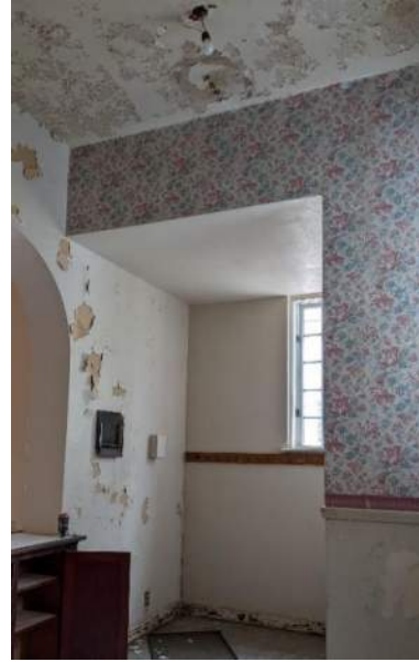
XAI.47 – Office 201. Damaged walls, ceiling, and wallpaper.
