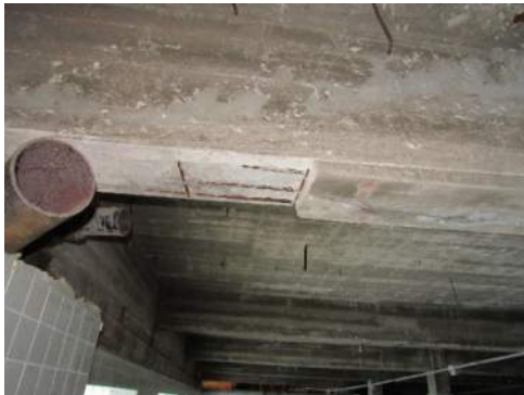
S.1 – Typical overhead beam repair due to original construction.
