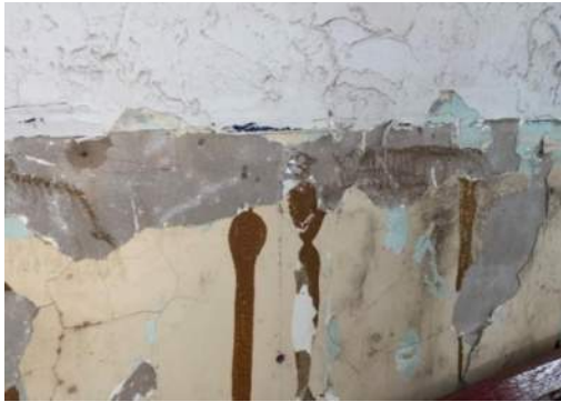
XAI.50 – Room 202. Damaged plaster.
