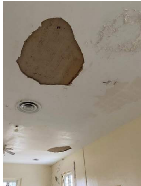
XAI.80 – Men's Bath 218. Damaged plaster in ceiling.
