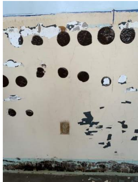
XAI.61 – Room 207. Damaged plaster wall and abandoned adhesive.
