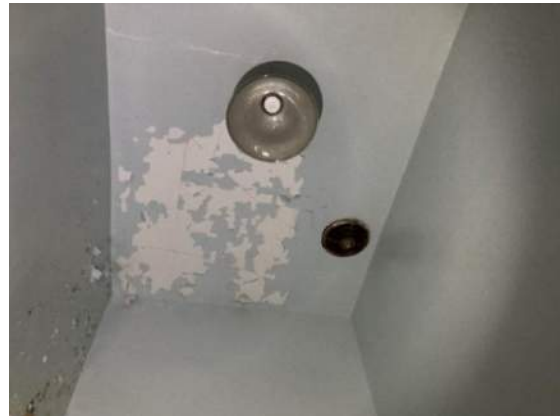
XAI.86 – Toilet 223. Damaged ceiling plaster.
