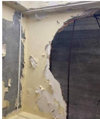
XAI.37 – Toilet 118. Damaged plaster ceiling.
