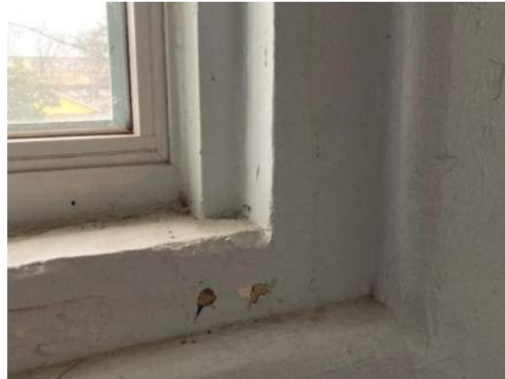
XAI.74 – Room 216. Damaged plaster at window.
