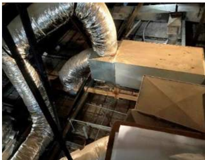
XM.1 Abandoned Blower Coil Unit
