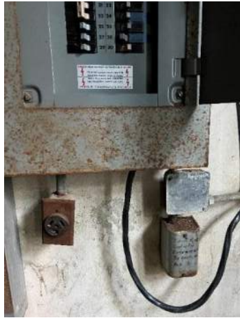
XE.7 Rust on Electrical Equipment
