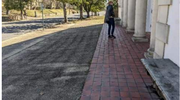
XC.5– Exterior at North. Quarry tile and damaged concrete at plaza.
