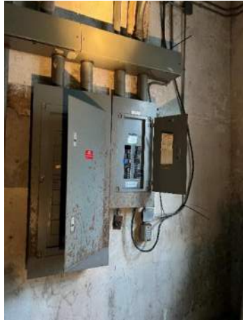
XE.8 Rust on electrical Equipment
