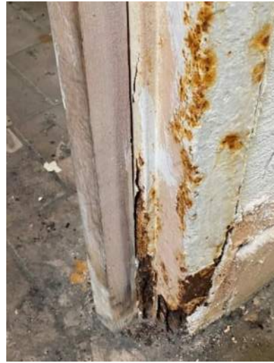
XAI.41 – Toilet 120. Damage at door frame.
