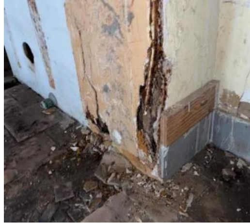
XAI.35 – Pool Room 117. Damaged wall plaster.
