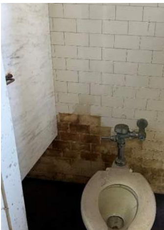
XP.3 Plumbing Fixture
