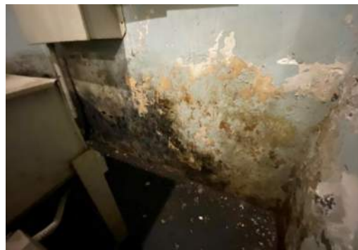
XAI.30 – Mechanical 115. Deteriorated plaster wall.
