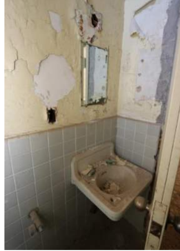
XAI.36 – Toilet 118. Damaged plaster walls.
