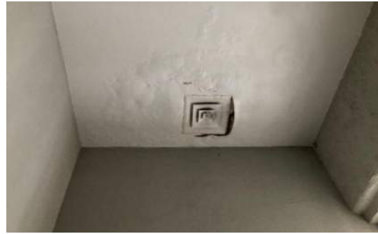
XAI.66 – Toilet 210. Damaged ceiling plaster.
