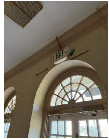
XE.10 emergency Light Fixtures
