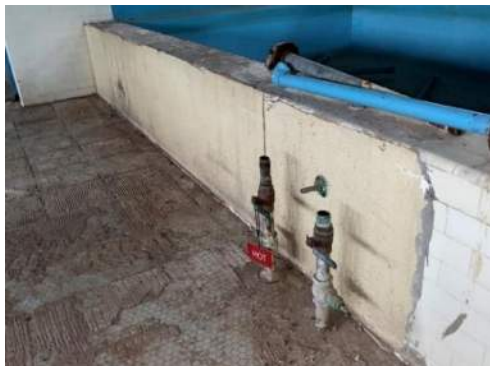
XAI.53 – Pool Room 203. Damaged wall and floor tile.
