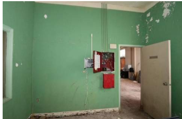
XAI.4 – Office 101. Existing alarm and damaged plaster.
