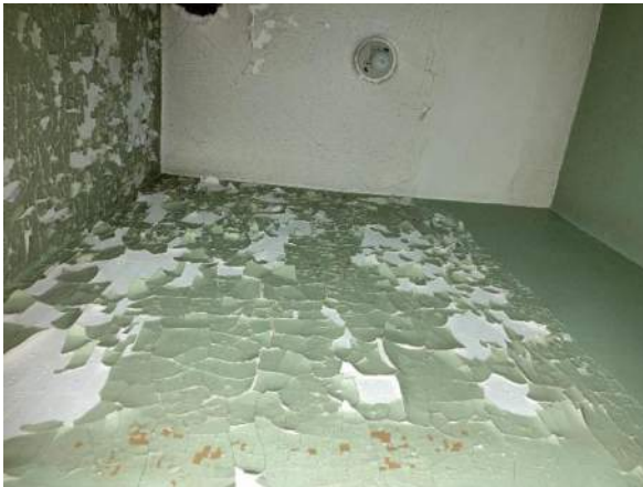
XAI.88 – Janitorial Closet 224. Damaged wall plaster.
