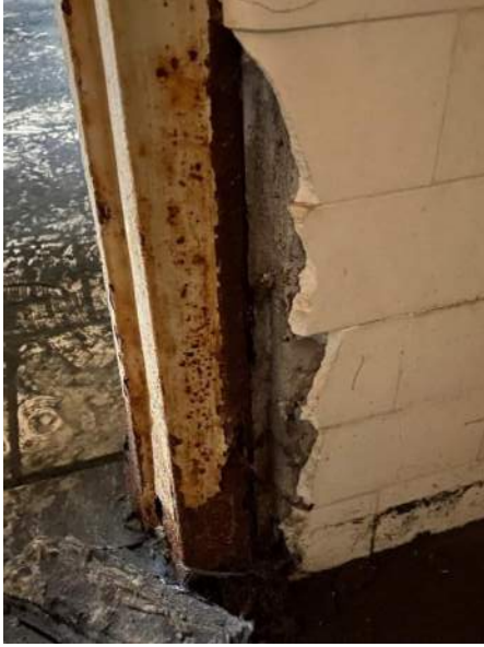
XAI.32 – Toilet 116. Damaged tiles and deteriorated door frame.
