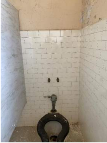
XAI.81 – Toilet 219. Damaged plaster and tiled walls, and plumbing.
