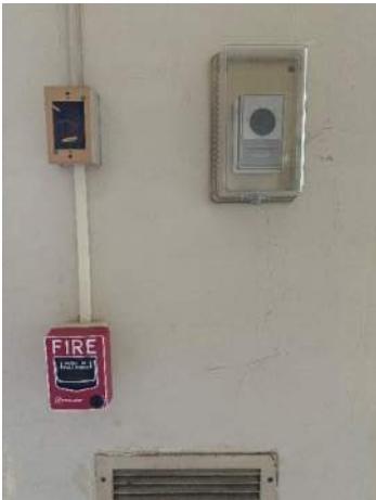
XE.23 Missing Fire Alarm Device
