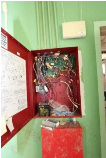
XE.1 Existing Fire Alarm System
