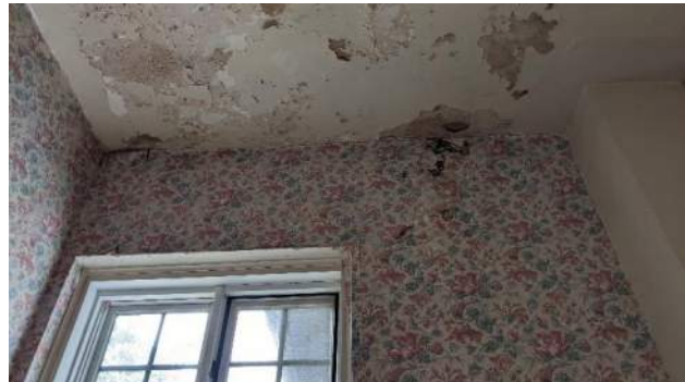
XAI.48 – Office 201. Damaged wallpaper and ceiling.
