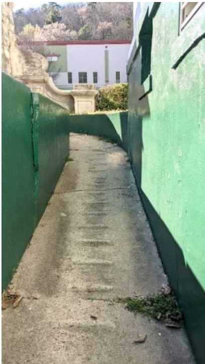
XAE.13 - Exterior at South. Deteriorated concrete ramp to basement and concrete retaining wall.
