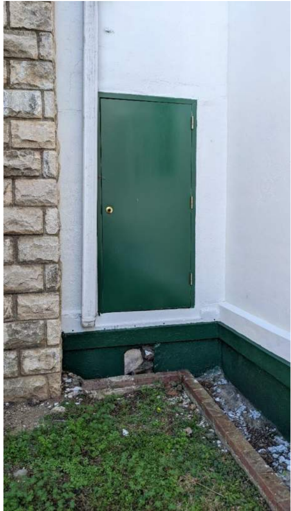
XAE.14– Exterior at North. Exit with no stair to grade.
