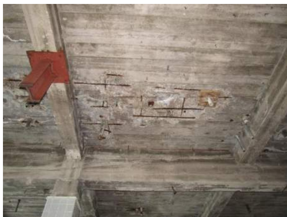
S.2 – Typical overhead slab repair area due to corrosion of reinforcing steel.
