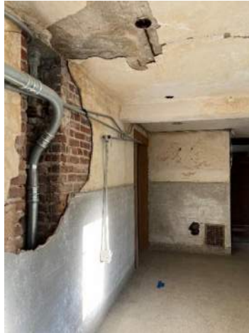
XE.37 Broken Conduit/Grounding System
