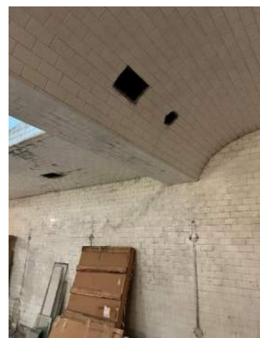
XE.14 Missing Light Fixture Openings
