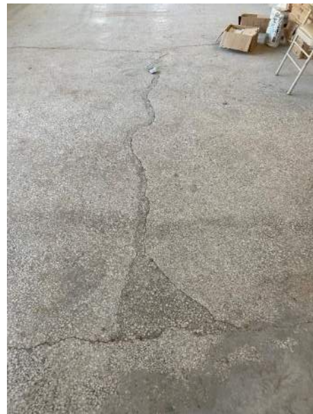
XA.74 – Men's Dressing 205. Detail of cracks in floor.
