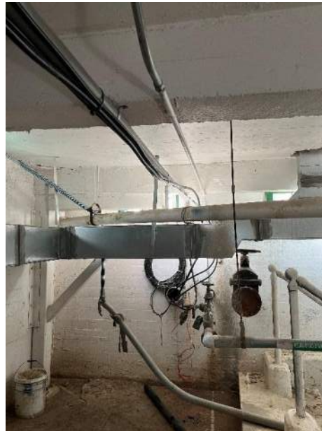
XF.1 Fire and Water Service
