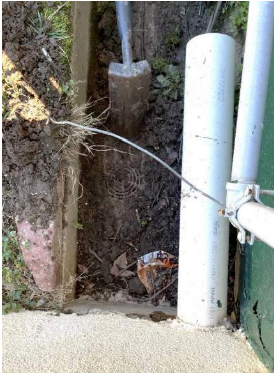
XAE.16 – Clogged drain in north side runnel. Note, the drainage (large white pipe) from the north side of the Sunporch roof also drains into this runnel.
