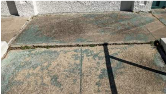
XAE.11– Exterior at West. Damaged ramp and landing at entrance.
