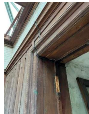
XE.6 Exposed Wiring
