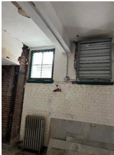
XE.20 Junction Box with Partial Cover Plate
