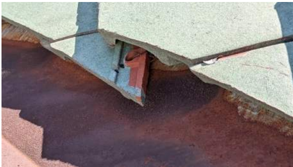
XAE.22 – Roof. Damaged green glazed vitrified clay roof tiles and copper flashing.
