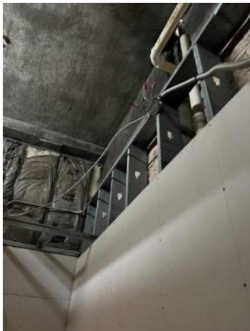
XE.36 Incomplete Open Wiring
