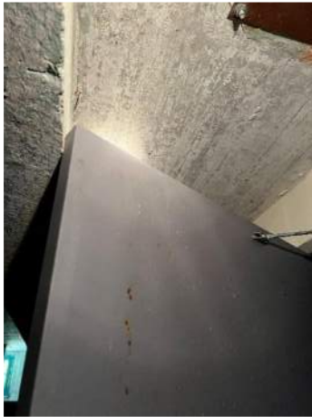
XE.26 Elevator Equipment Entry Door
