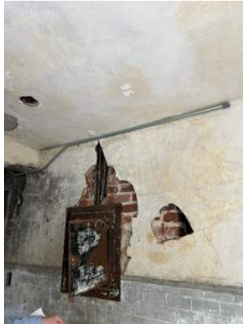
XE.39 Broken Conduit/Grounding System
