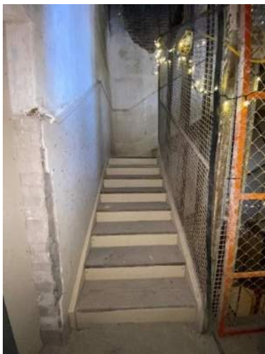
XA.83 – Stair Hall 216. Looking south. Note the wood treads on the stairs.
