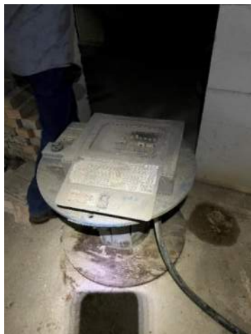
XE.9 Temporary Wiring and Distribution
