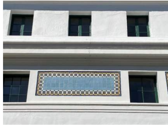
XAE.8 – Exterior. Damaged tile, cornice, and wall.
