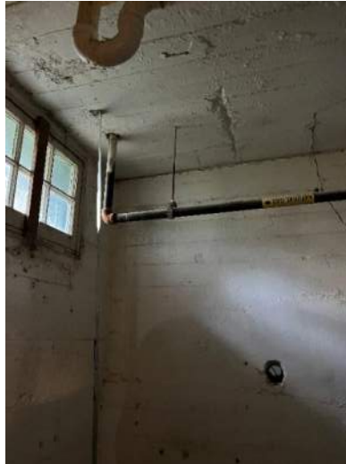
XP.4 Existing Gas Piping
