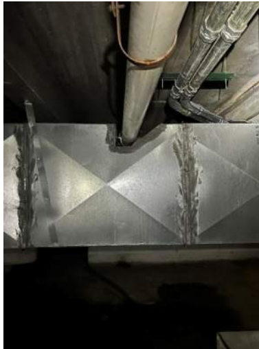
XM.3 Existing Ductwork
