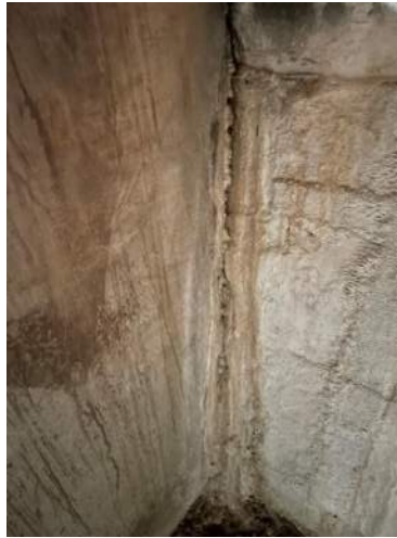
XP.11 Springs Collection Basin Leak
