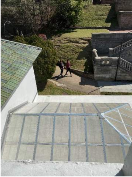
XAE.20 – Skylight. Deteriorated to be replaced.
