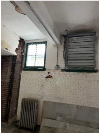
XE.16 Junction Box with Partial Cover Plate
