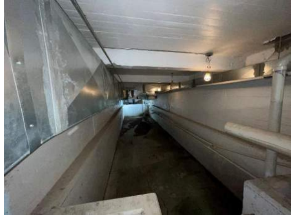
XA.4 – B10 Pool – Typical conditions at pool with roof drains into pool and ductwork overhead.
