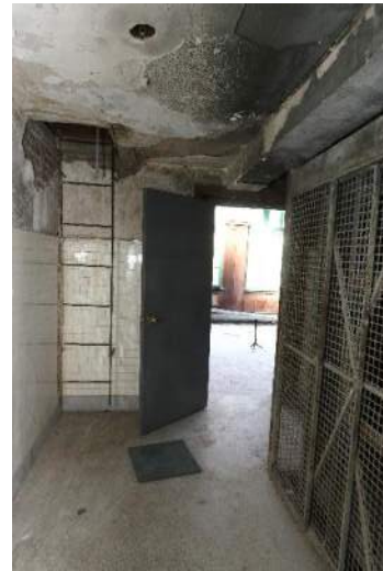
XA.91 – Men's Stair 303. Looking west. Note the ladder on the wall is the roof hatch.
