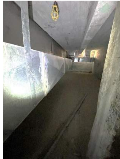
XA.16 – B13 Typical low ductwork in basement.
