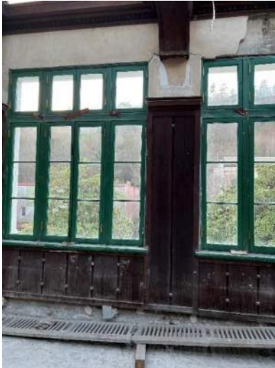
XM.8 Abandoned Radiator
