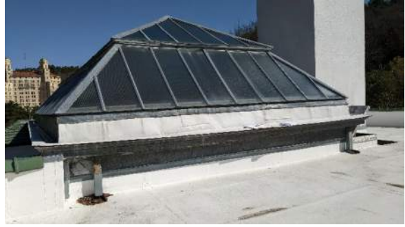
XAE.23 – Skylight. Deteriorated to be replaced.
