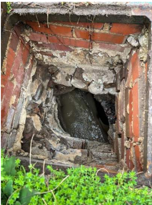
XAE.17– Access to Display Spring drainage at NE of building.
