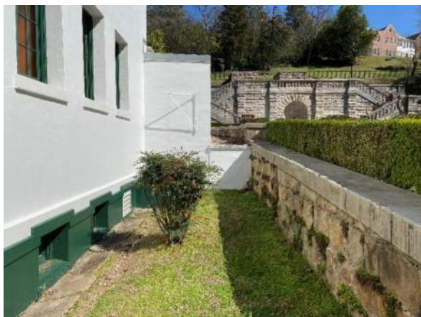
XAE.15 – Exterior at South. Deteriorated stone retaining wall and concrete runnel.
