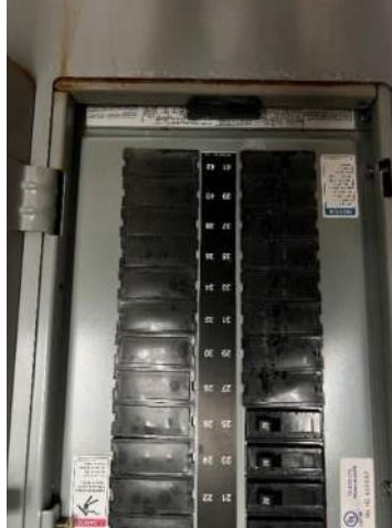
XE.28 Rust on Electrical Equipment
