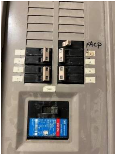
XE.1 Existing Panel with FACP CB in Off position
