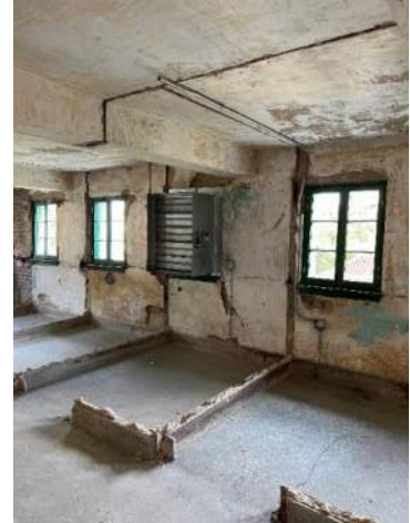
XE.40 Broken Conduit/Grounding System
