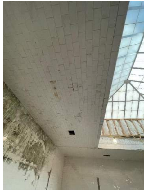
XA.50 – Men's Bath Hall 113. Detail of stained wall tiles and tiled ceiling.
