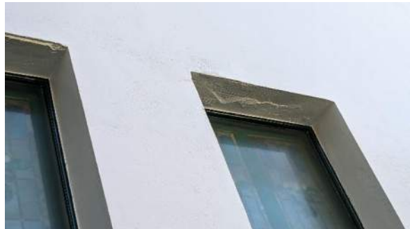
XAE.9 – Windows. Damaged plaster.
