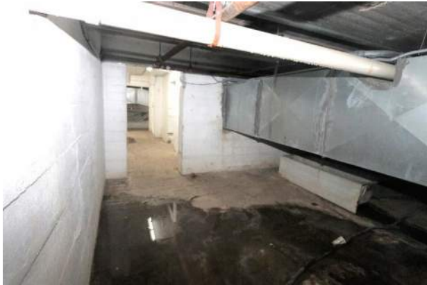
XA.2 – Basement B01 – Typical Conditions in east rooms with standing water and low head-height at ductwork in basement.
