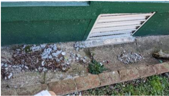
XAE.12– Exterior at North. Damaged runnel and louver.
