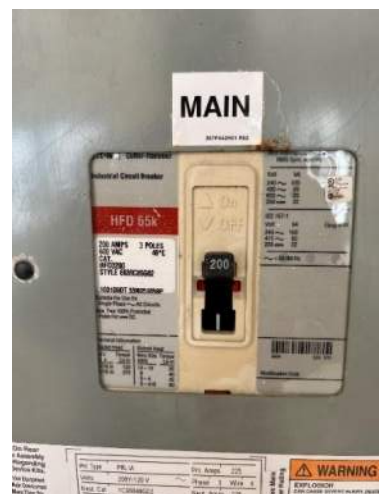
XE.41 Rust on Electrical Equipment
