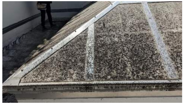
XAE.25 – Northeast skylight staining from berries from tree above roof.
