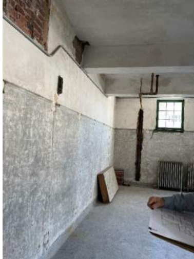
XM.9 Abandoned Steam Piping
