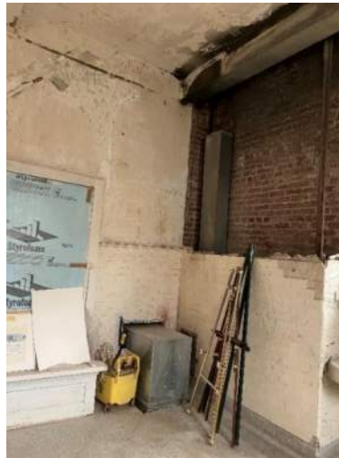
XM.10 Abandoned Ductwork
