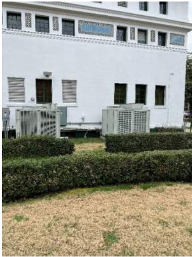
XM.1 Hale and Maurice Condensing Units
