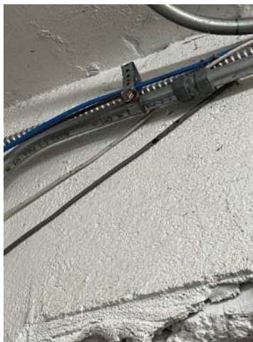
XE.21 Ground Connection
