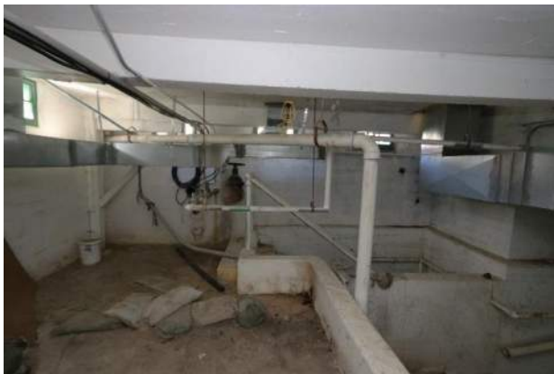
XA.3 – B10 Pool. Typical conditions at south end of pool with utilities, structural stabilization steel, and low ductwork.
