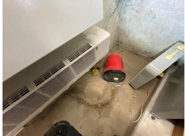
XA.15 – B22 Blocked floor drain in elevator machine room.
