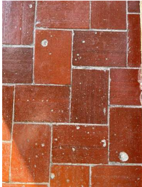
XA.33 – Sunporch 109. Damaged mosaic border and base to be replaced.
