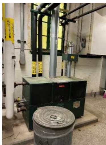
XM.4 Existing Boiler
