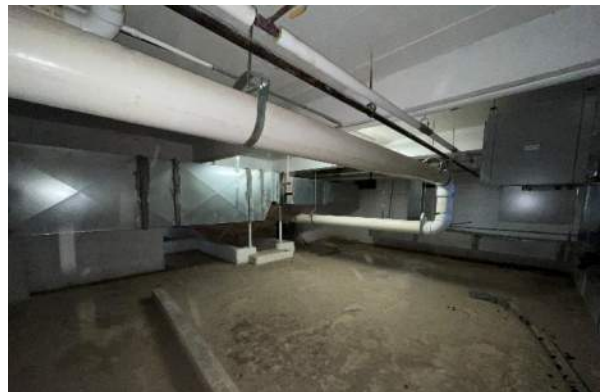
XA.5 – B10 Pool Deck – Typical conditions at pool deck with low ductwork, piping, and equipment. Note, the ductwork is over the entrance stairs into the pool.
