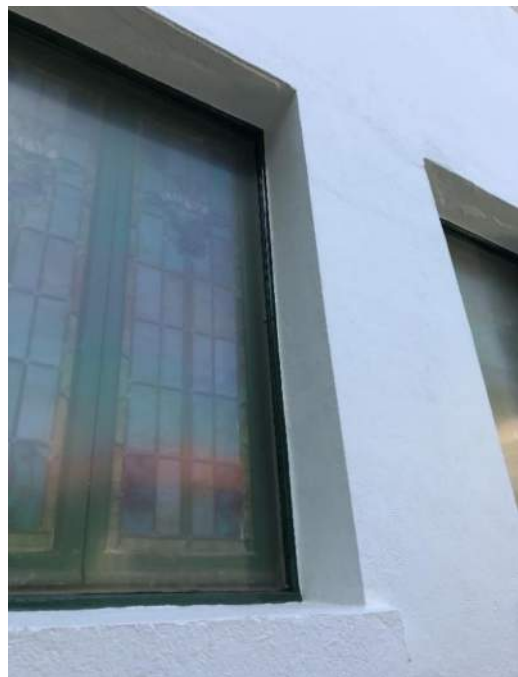
XAE.19 – Yellowed plexiglass coverings over historic stained glass windows. Coverings are not properly vented.
