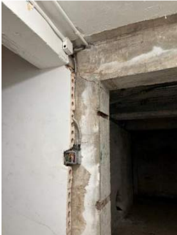
XE.34 Missing Cover Plates
