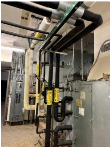
XM.2 Existing Air Handling Unit
