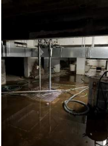
XP.10 Springs Flooding Basement
