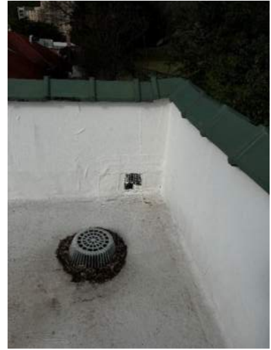
XP.5 Roof Drain
