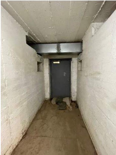
XA.8 – B11 Hall with low overhead ducts and door to the exterior ramp. Note the sandbags in the door opening.
