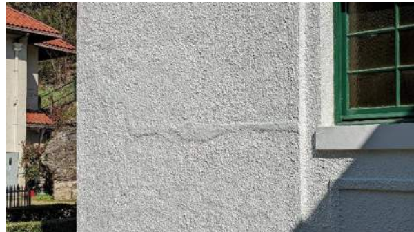
XAE.7 – Exterior. Patched stucco where previously cracked.
