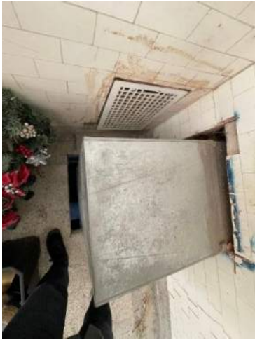
XA.63 – Men's Massage Room 116. Duct through floor and wall.
