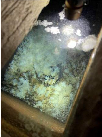
XA.13 – B01 Clogged hot spring water cistern.
