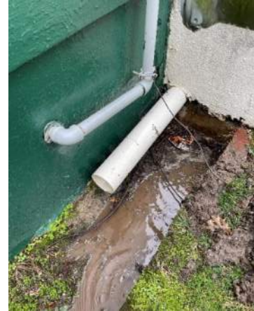
XP.13 Silted Up Runnel Drain
