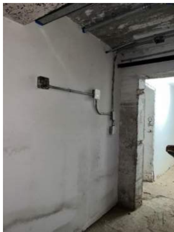
XE.18 Junction Box with Missing Cover Plate
