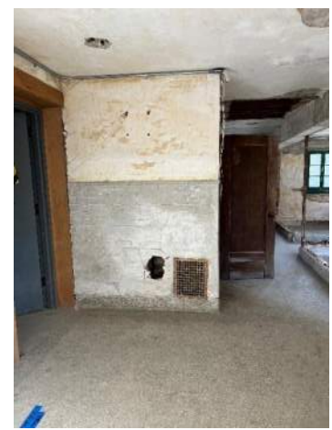
XE.15 Junction Box with Missing Cover Plate
