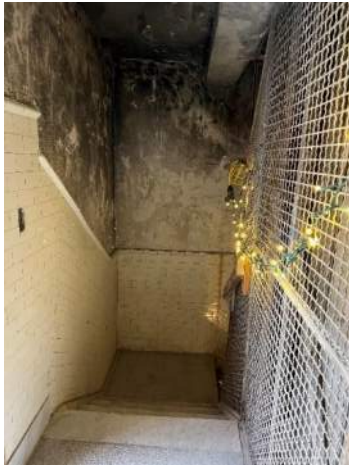
XE.7 Temporary Lighting
