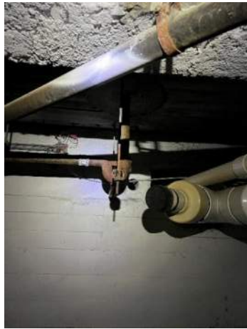
XE.17 Junction Box with Missing Cover Plate
