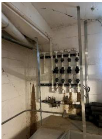
XP.12 Existing Irrigation System
