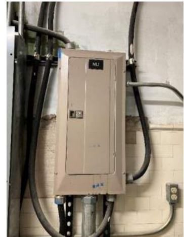
XE.13 Panel for Temporary Service
