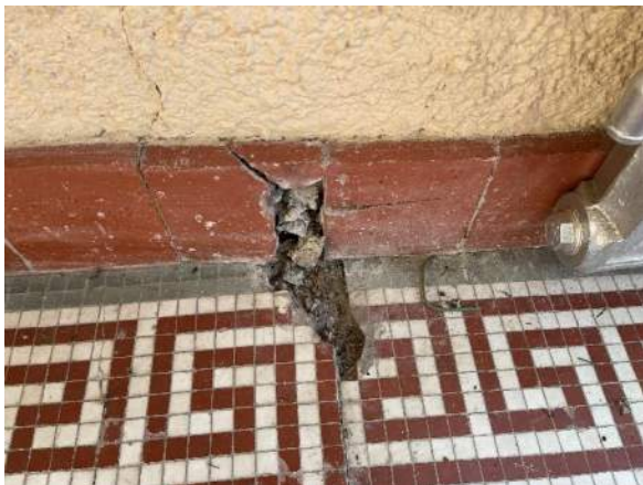
XA.32 – Sunporch 109. Damaged mosaic border and base to be replaced.
