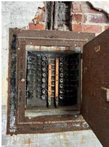
XE.3 Existing Panelboard to be Removed
