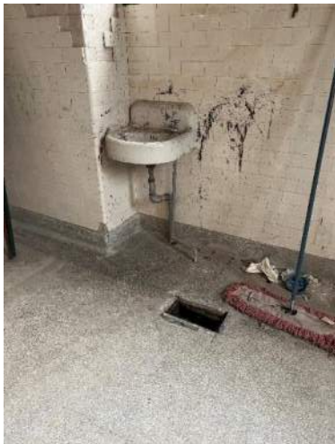
XP.9 Existing Plumbing Fixture
