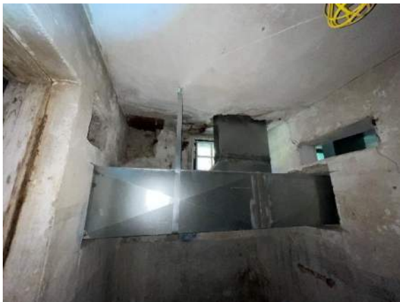
XA.14 – B15 Typical low ductwork.
