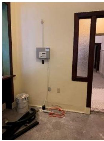
XE.11 Existing Security System
