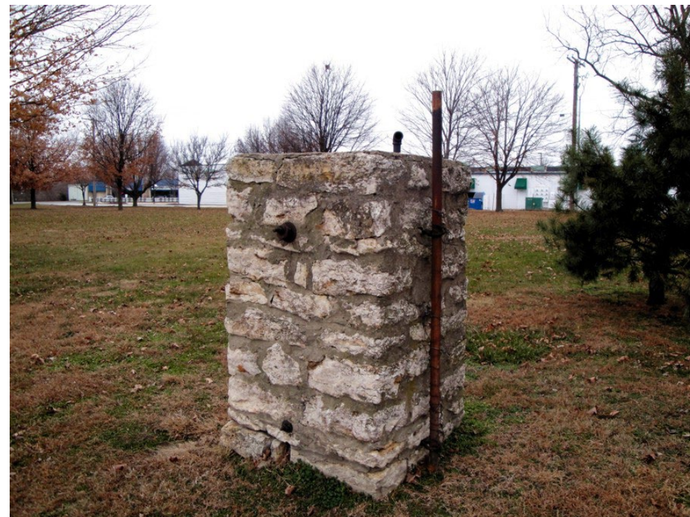
The stone post located in the front yard near the wayside sign (Jackson/NPS 2009).
