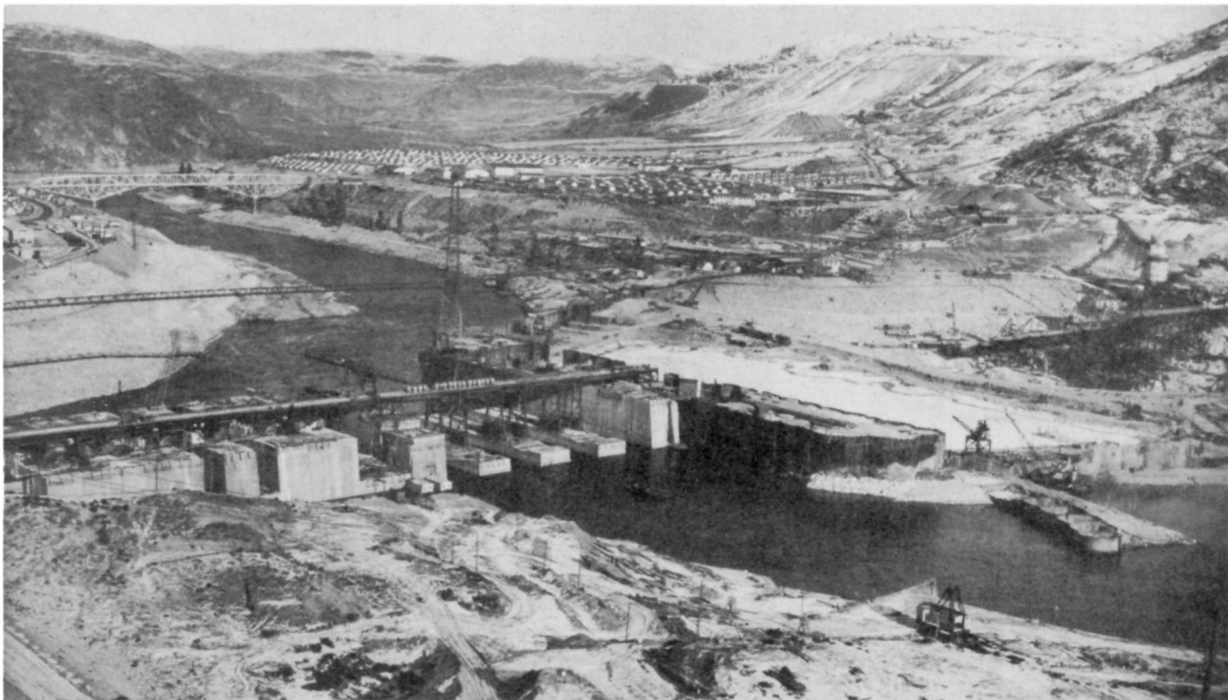
COLUMBIA RIVER DIVERTED. VIEW FROM WEST BANK SHOWS DIVERTED RIVER FLOWING THROUGH GAPS IN FOUNDATION. NORTH AND SOUTH COFFER DAMS SHUT OFF THE OLD RIVER BED. THE WATER IN OLD RIVER BED WILL BE PUMPED OUT AND OVERBURDEN EXCAVATED. TWO EAST TRESTLES WILL BE EXTENDED TO POUR CEMENT IN OLD RIVER BED. WEST SIDE COFFER DAM IS BEING DISMANTLED
