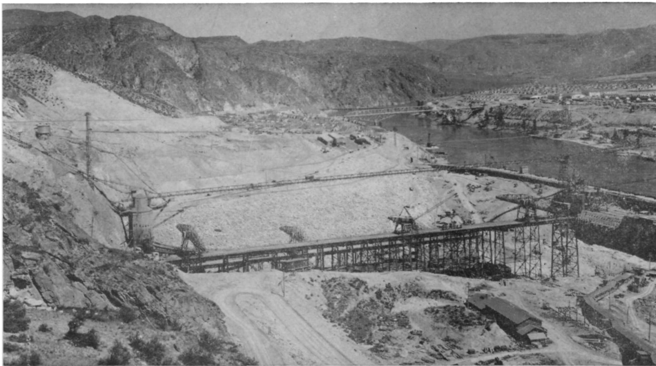
Photo by Bureau of Reclamation Panoramic view of Grand Coulee Dam construction. Upper plate shows West side with Engineers Town in background. Lower plate shows East side construction.
