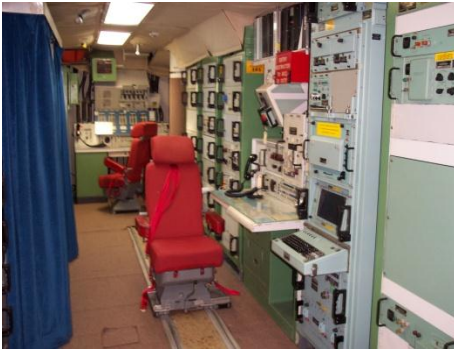
Launch Control Center Delta-01
