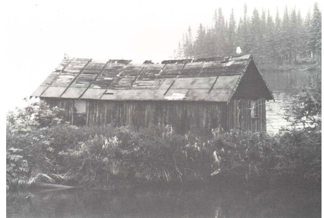
View of the Net House (now in ruins) from the inner harbor, ca. 1985 (Bradford for NPS).
