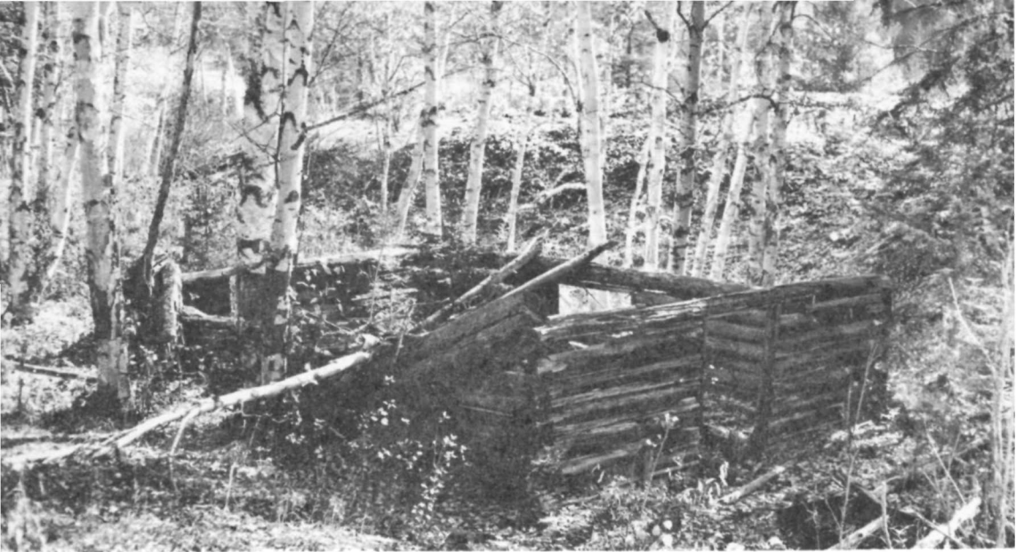
Minong Mine blacksmith shop, today roofless and disintegrating, located near the mine.
