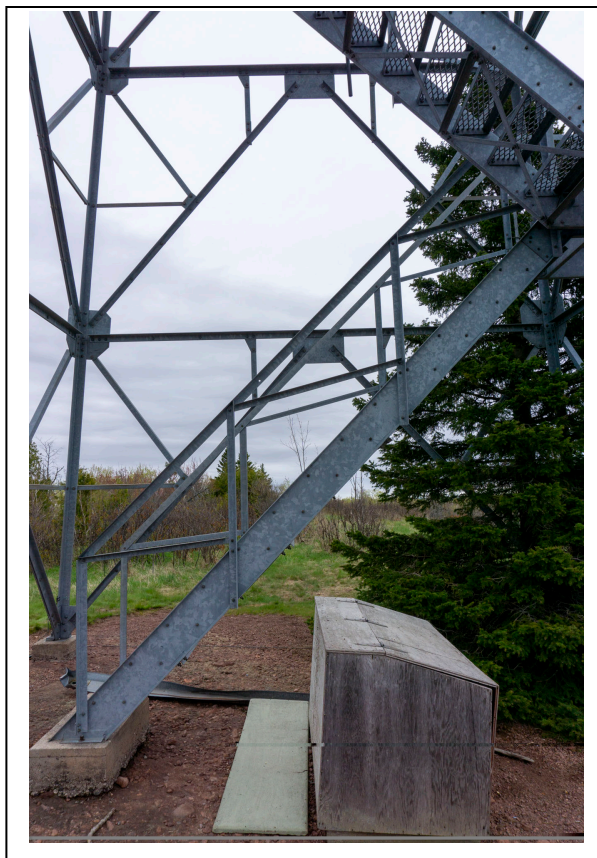
Figure 6: Bottom stair run at New Feldtmann Fire Tower, showing stair and tower construction, looking east. Photo by Natalie Young, 2019.
