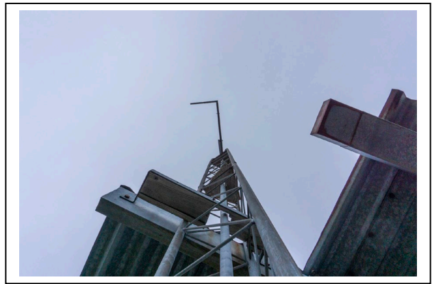
Figure 12: Top of radio antenna protruding above roof at New Feldtmann Fire Tower, looking southwest. Photo by Natalie Young, 2019.
