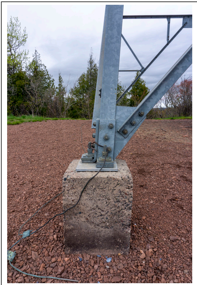
Figure 4: Concrete foundation pier with grounding for lightning protection at New Feldtmann Fire Tower, looking south. Photo by Natalie Young, 2019.
