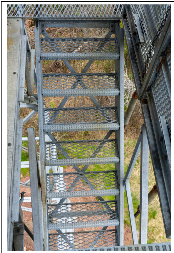
Figure 7: Top stair run at New Feldtmann Fire Tower, showing expanded metal stair treads, looking north. Photo by Natalie Young, 2019.
