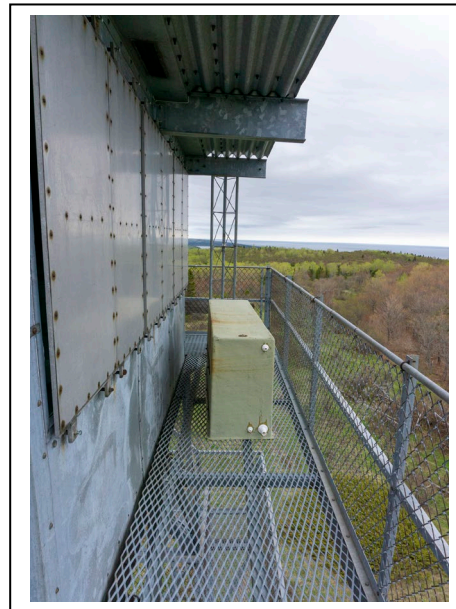
Figure 14: Balcony with container of unknown purpose at New Feldtmann Fire Tower, radio antenna in background, facing east. Photo by Natalie Young, 2019.
