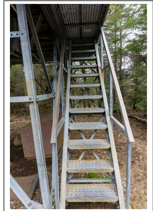
Figure 8: Metal stairs at Ishpeming Fire Tower, 2019, looking W. Photo by Natalie Young.
