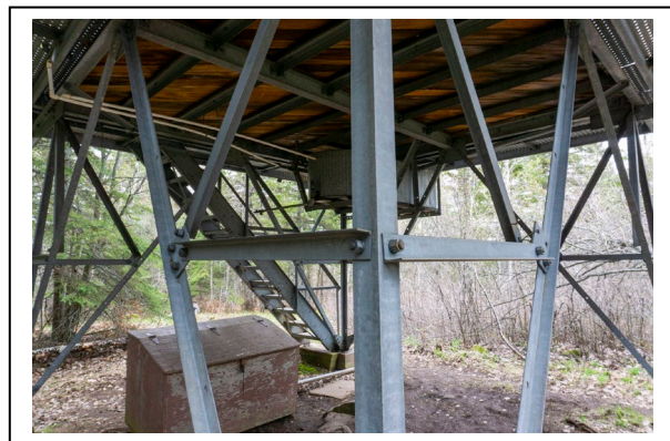
Figure 4: Angle steel construction of Ishpeming Fire Tower, 2019, looking NE. Photo by Natalie Young.
