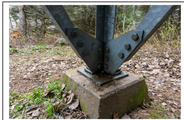
Figure 6: Connection of steel tower to concrete foundation piers, 2019, looking SE. Photo by Natalie Young.
