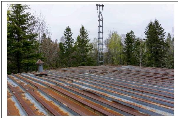
Figure 18: Ishpeming Fire Tower roof with vent, 2019, looking NE. Photo by Natalie Young.
