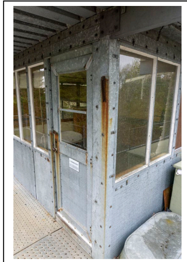
Figure 16: Metal entrance door on south side of Ishpeming Fire Tower cab, 2019, looking NW. Photo by Natalie Young.
