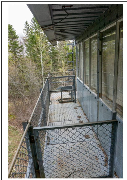
Figure 11: Chain link fencing around perimeter of balcony at Ishpeming Fire Tower, 2019, looking SE. Photo by Natalie Young.
