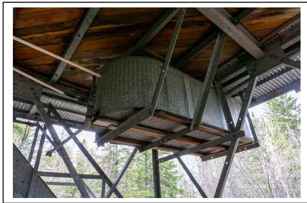
Figure 24: Corrugated metal container beneath Ishpeming Fire Tower cab floor, 2019, facing NE. Photo by Natalie Young.
