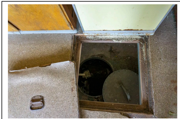
Figure 21: Opening to water tank below floor of Ishpeming Fire Tower cab, 2019, looking N. Photo by Natalie Young.
