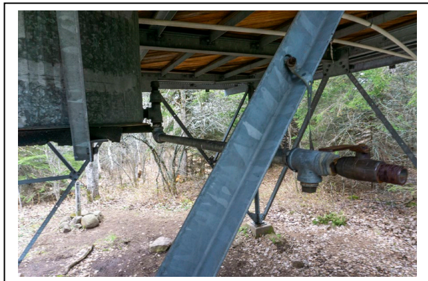
Figure 26: Metal piping from container below Ishpeming Fire Tower cab floor, 2019, looking NW. Photo by Natalie Young.
