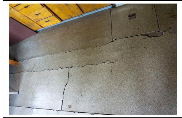
Figure 19: Rolled flooring of Ishpeming Fire Tower cab, 2019, looking N. Photo by Natalie Young.
