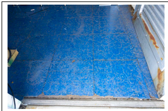
Figure 26: Ojibway Fire Tower cab floor tiles at entrance, facing north. Photo by Natalie Young, 2019.
