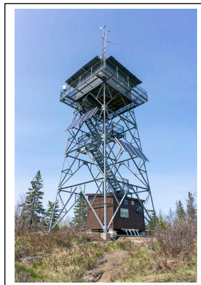
Figure 10: Solar panels on south and west sides of Ojibway Fire Tower, looking northeast. Photo by Natalie Young, 2019.
