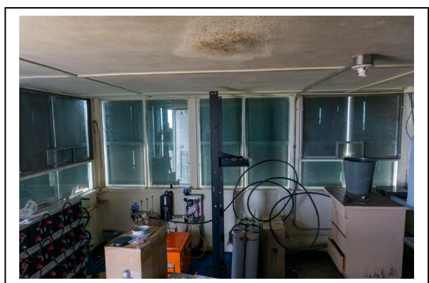
Figure 33: Interior of Ojibway Fire Tower cab, looking west. Photo by Natalie Young, 2019.
