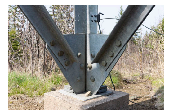
Figure 9: Ojibway Fire Tower foundation pier with structural members bolted together. Grounding wire behind. Photo by Natalie Young, 2019.
