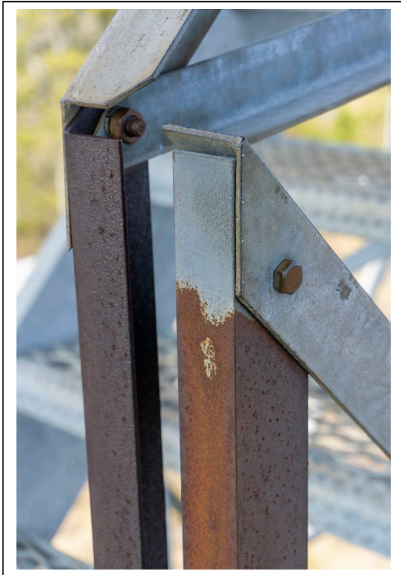
Figure 17: Detail of handrail construction on Ojibway Fire Tower stairway. Photo by Natalie Young, 2019.
