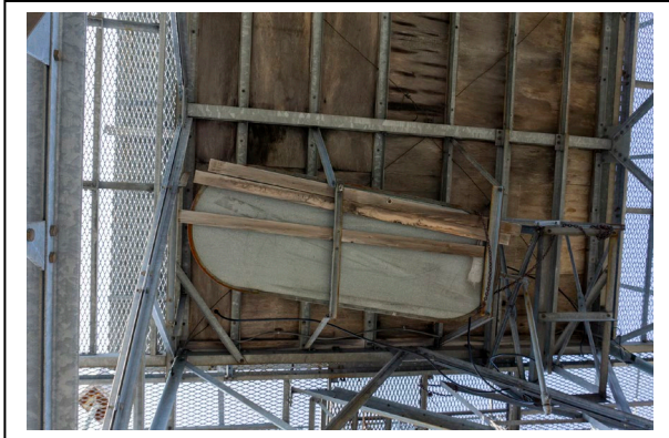
Figure 28: Position of metal water tank beneath floor of Ojibway Fire Tower cab, looking north (looking up). Photo by Natalie Young, 2019.
