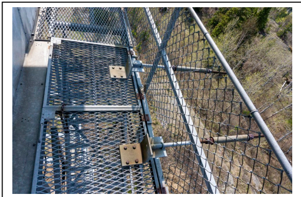
Figure 19: Ojibway Fire Tower balcony hatch with cantilevered weights, looking west. Photo by Natalie Young, 2019.
