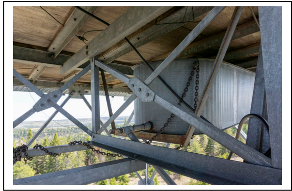
Figure 29: Metal water tank beneath floor of Ojibway Fire Tower cab, looking northwest. Photo by Natalie Young, 2019.
