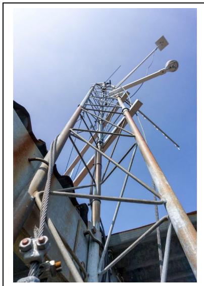
Figure 21: Ojibway Fire Tower radio antenna on southwest corner of balcony, looking northeast. Photo by Natalie Young, 2019.
