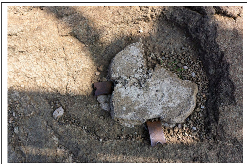
Figure 38: Typical embedment in rock at Ojibway Fire Tower. Purpose of these is unknown, but they may have been used as tie-downs for guy wires for the tower or the associated antennae. Photo by Natalie Young, 2019.
