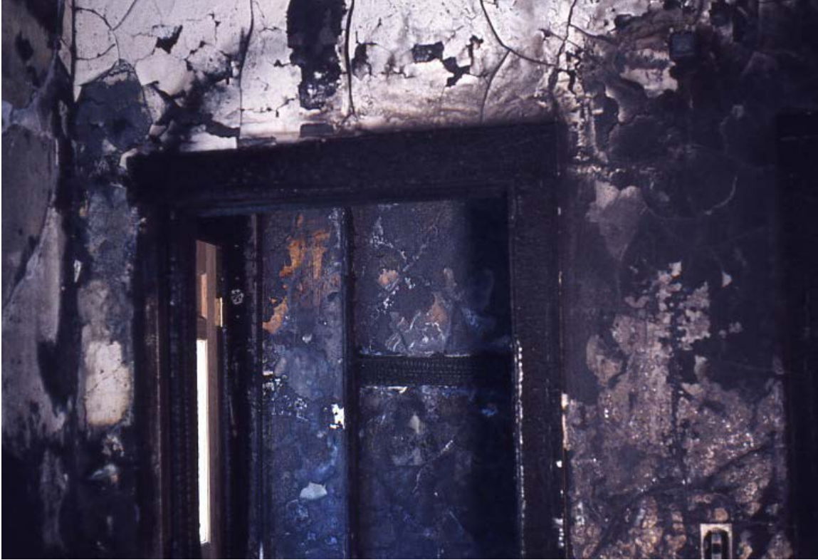
Figure 9. 1975 fire damage in the kitchen and back hall. JOFI 1504, Box 10, Folder 12, NPS, 1975.
