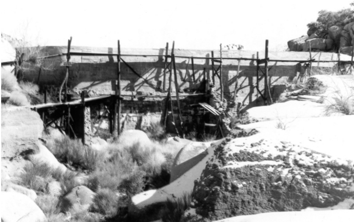
History #4: Construction of primary Keys Ranch Dam, looking east. (Joshua Tree National Park archives, accession #531-I2242, Ross Holland, 1971)
