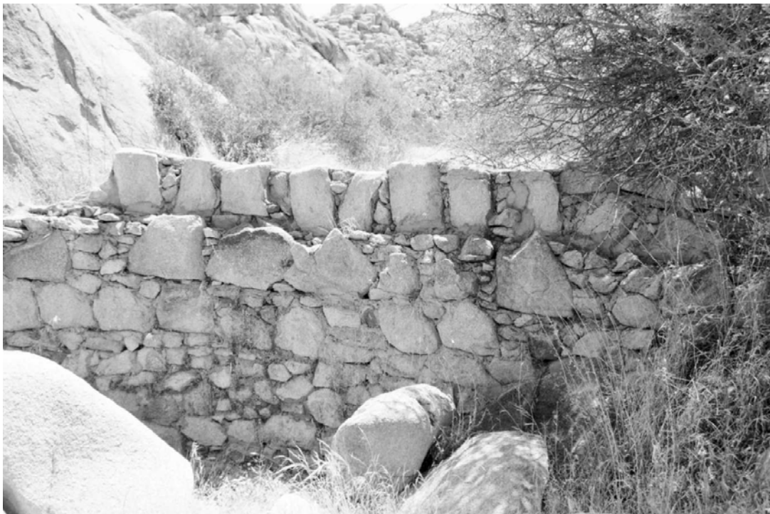
Buildings and Structures #13: Cow Camp retaining wall associated with agricultural area, looking south. (PGSO, CLI negative #JOTR-N-0003-9, 1999)
