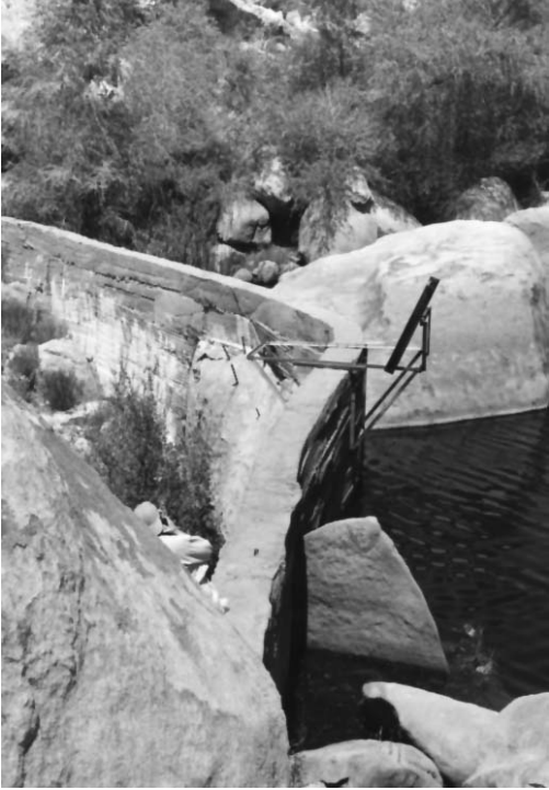
Buildings and Structures #14: Cow Camp dam from above, looking north. (PGSO, LCS, 1992)
