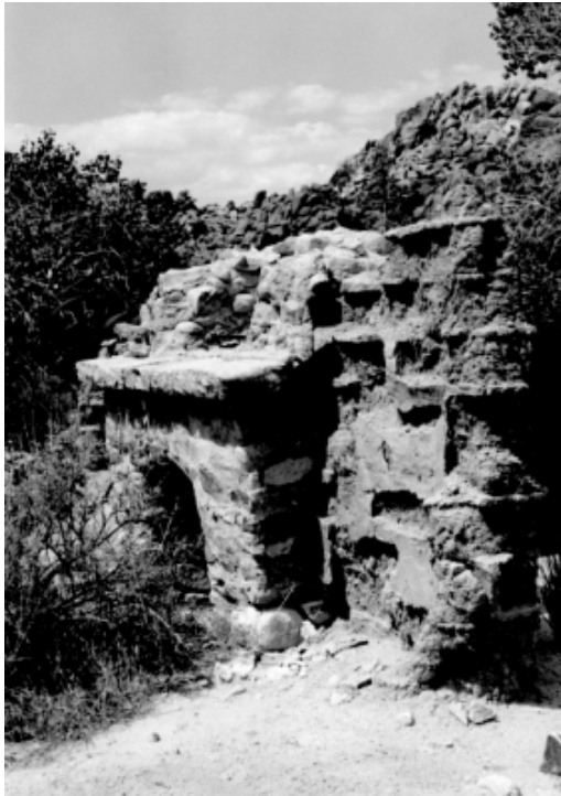
Small Scale Features #2: Desert Queen Ranch adobe ruin with fireplace, looking north. (PGSO, LCS, 1992)
