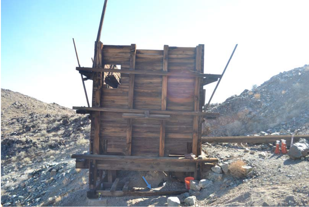
Figure 5: Bin #1, looking east. Decay at the south sill (just out of view) has allowed the ore bin to rotate out of plumb to the south. Also, note the condition of the timber spreader between the north and south sill (bottom center).
