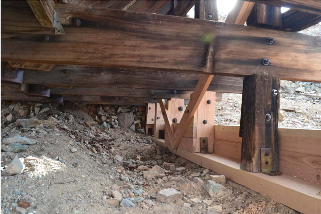
Figure 11: Ore bin #2, following replacement of west sill, column extensions, splints, and diagonal bracing. Note boarding installed to isolate the sill and column bases from soil (right).
