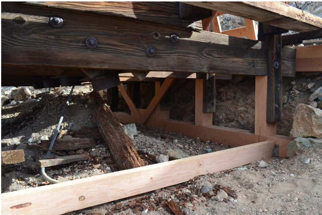
Figure 8: Ore bin #1 after installation of replacement column extensions, south sill, diagonal bracing, and spreader (foreground). Original splints were salvaged for reinstallation. Holes bored for borate rod installation are visible at the base of each column extension.
