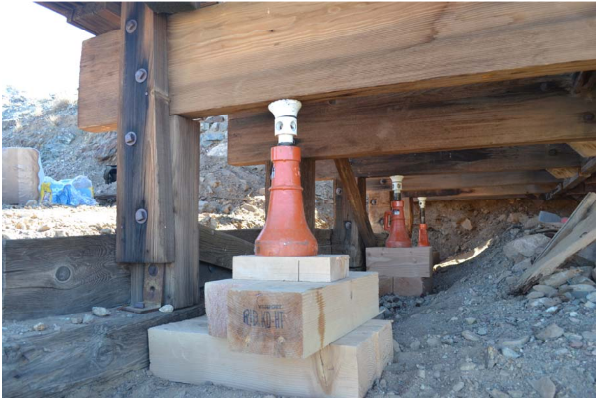
Figure 7: Cribbing and screw jacks were used to plumb Bin #2 (west) prior to removal of deteriorated sills and column extensions for repair or replacement.
