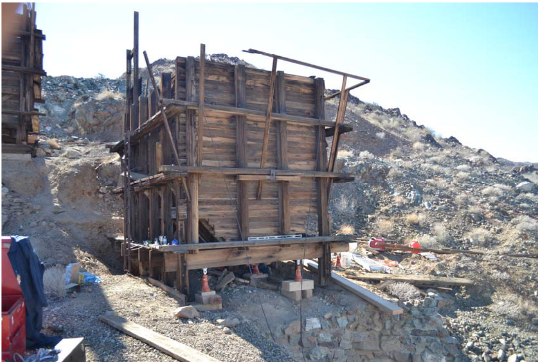
Figure 9: West ore bin supported on cribbing and screw jacks. New timber sill (right) is ready for installation on the west elevation.
