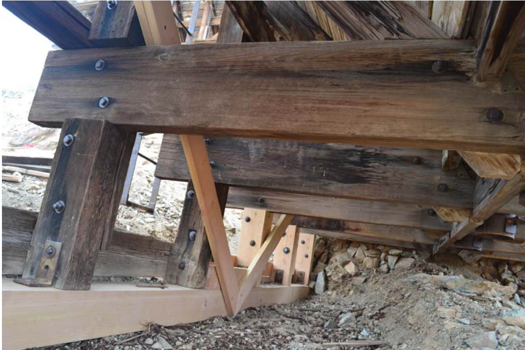
Figure 10: Ore bin #2, following replacement of east sill, column extensions, and diagonal bracing (left).
