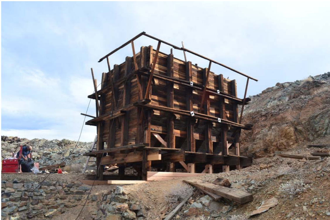
Figure 12: West ore bin with repairs completed, looking southeast. Note replacement boards attached to column extensions and intended to isolate substructure from soil (foreground).
