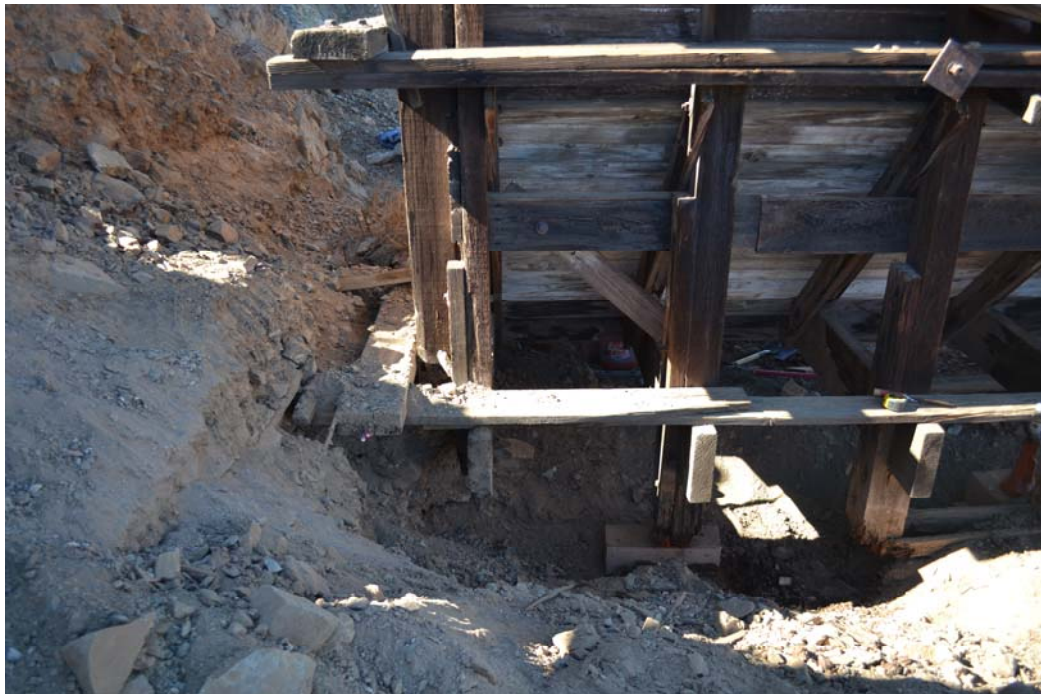
Figure 6: Bin #2, looking west. Note the condition of the east sill at its south end (bottom left, foreground). The sill and column extensions have completely decayed allowing the tipple to rotate out of plumb to the south.
