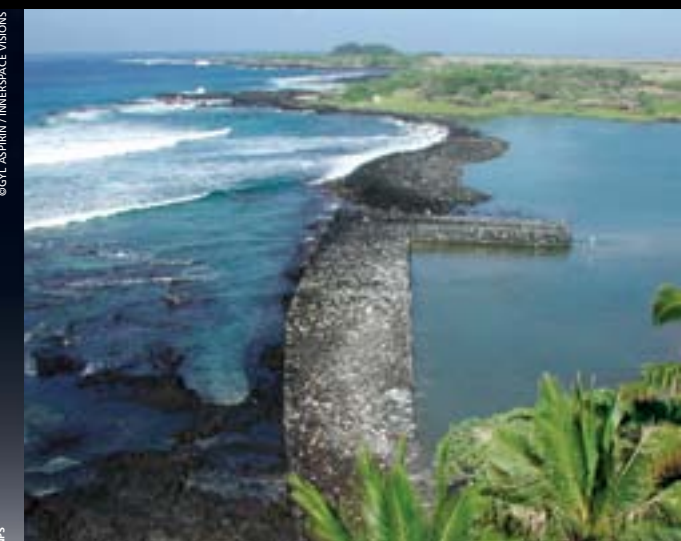
The kuapā, or rock wall, now being reconstructed, separates Kaloko fishpond from the ocean.
