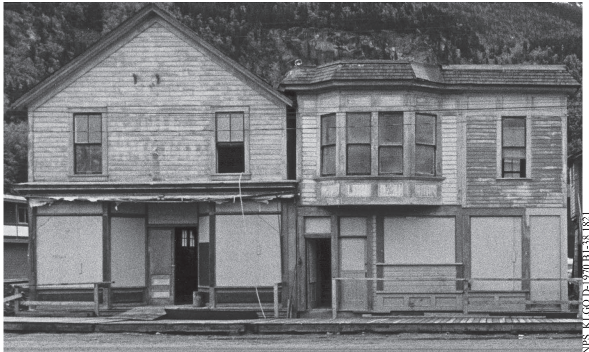
Mascot Saloon, Pacific Clipper Line Office, and Hern Liquor Store Prior to National Park Service restoration, 1977
