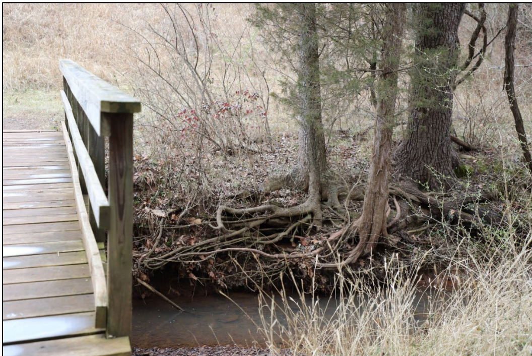
Fig. 20: View of wood bridge along the Second Manassas Trail and observed stream bank erosion along Chinn Branch (NCR CLP 2023).
