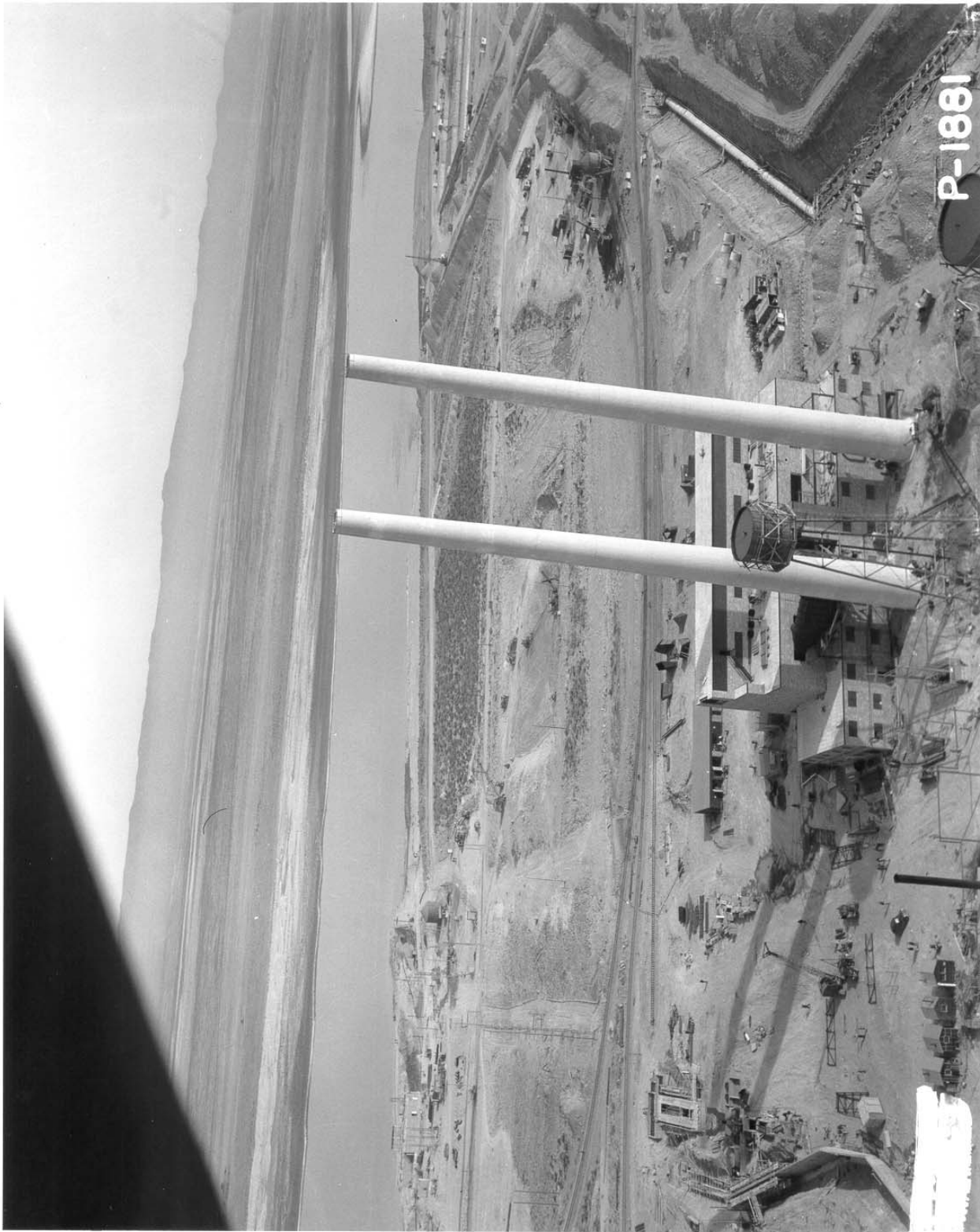
Photograph 24: The 184-B Power House under construction, viewed to the northeast in March 1944. The sewer line exiting to the Columbia river was used mainly for effluents from back-washing the filter basins. A separate Process Sewer Line (out of the picture to the right) for cooling water leaving the pile went to the 107-B Retention Basin, and ultimately to the river. [P-1881]
