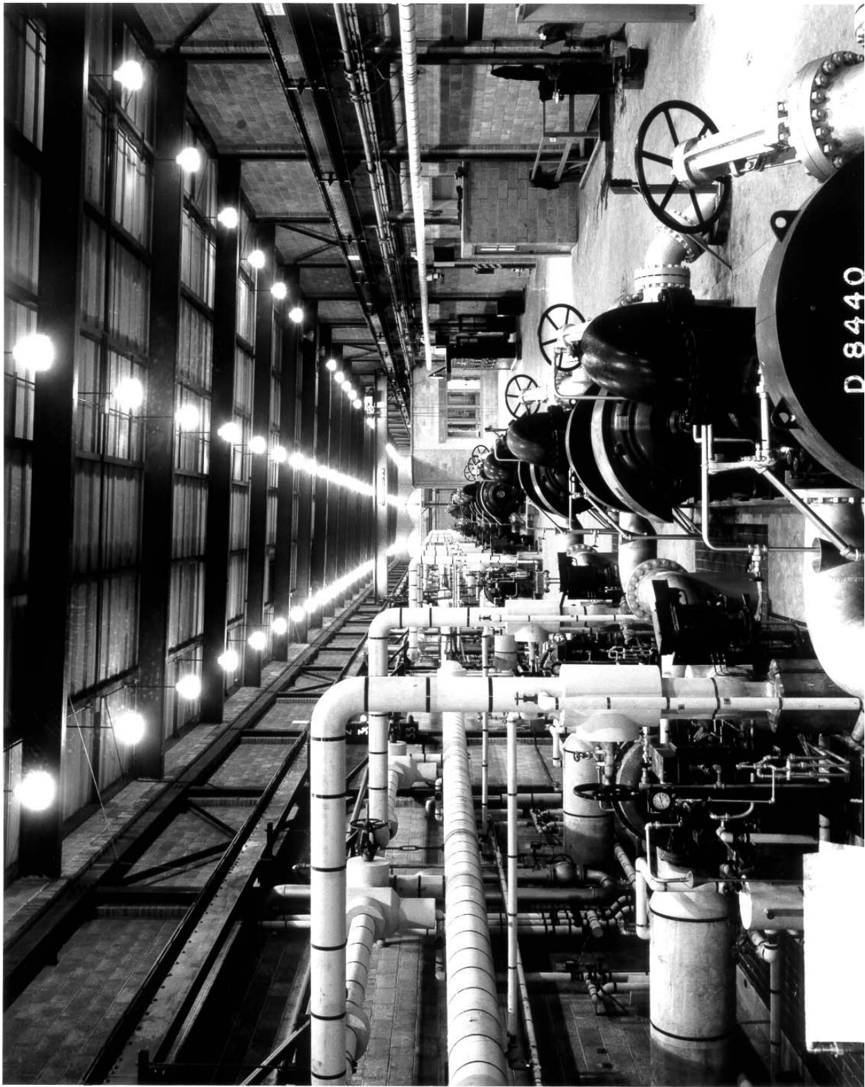
Photograph 19: Interior of the 190 Process Pump House, in this case in the 100-F Area in February 1945. Steam-driven pumps are on the left and electrically-driven pumps are on the right. [D-8440]
