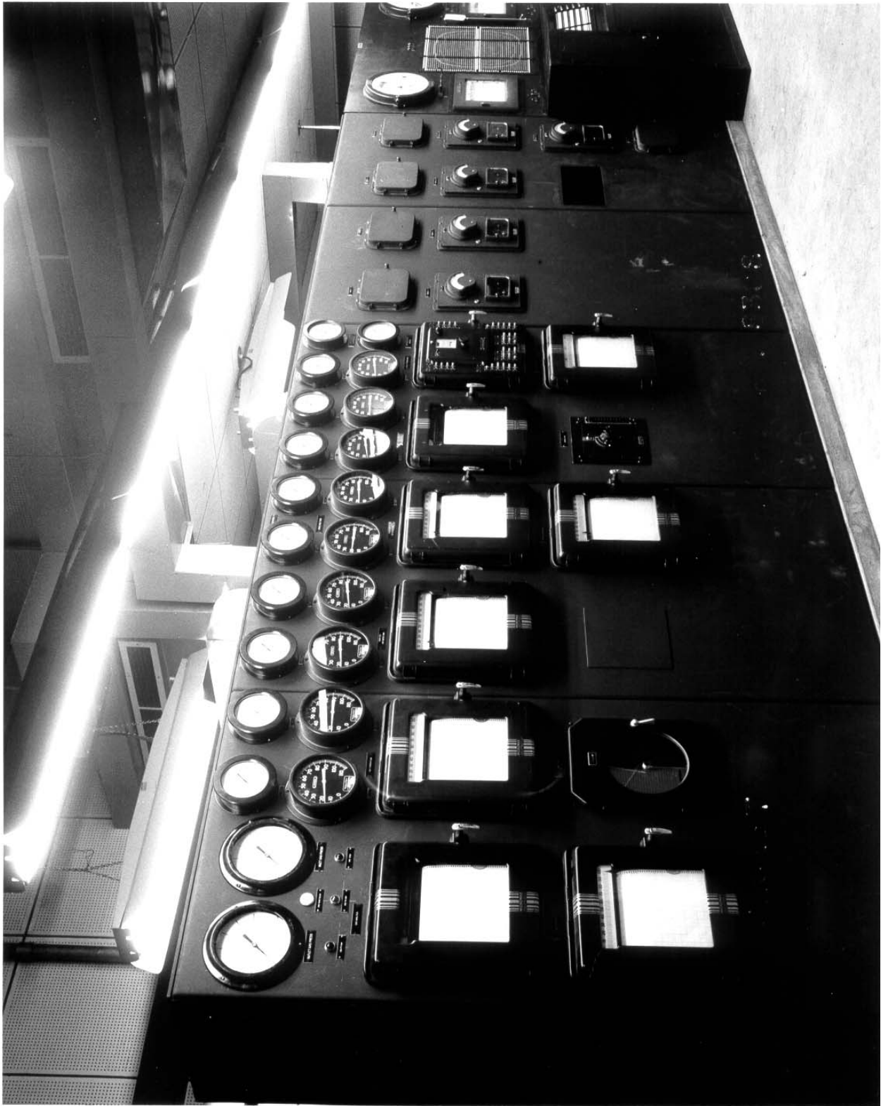
Photograph 30: Miscellaneous gauges and recorders on the wall opposite the Panellit gauges in a typical control room, 105-F Reactor in this case in February 1945. The temperature recorder for the 2,004 process tubes is at the far right side. [D-8308]
