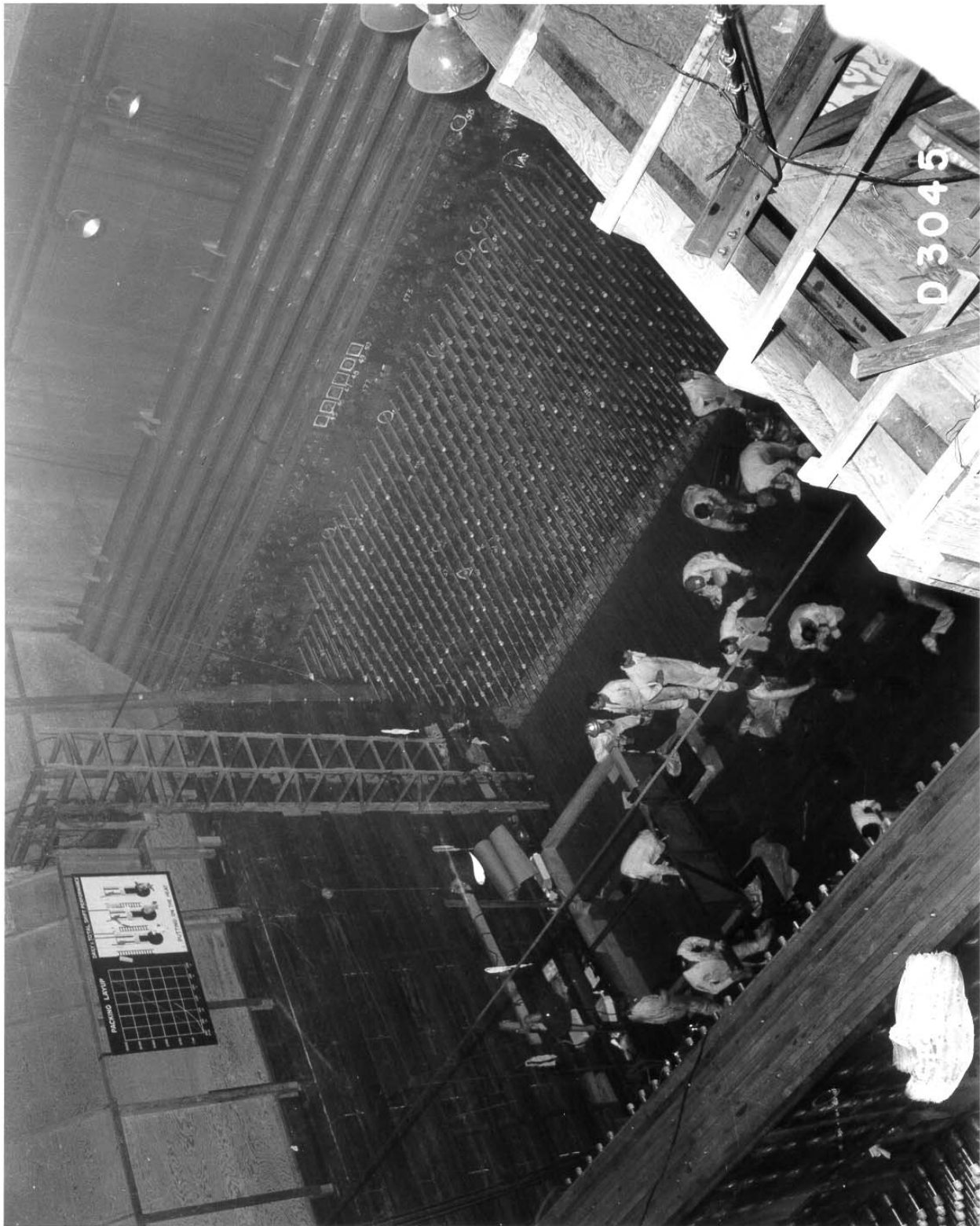
Photograph 6: Workers laying up the graphite core of the 105-B pile. In the lower-left can be seen a portion of the rear face of the pile, the top of its shielding wall, and the gun barrels protruding through it. The inside of the front face of the pile and its gun barrels can be seen toward the upper-right side. The angled top of the front shielding wall can be seen in the picture. All four walls were “stepped” in this manner where they joined with another wall or the ceiling to form a “labyrinth” joint, so that radiation would not have a straight route through any gaps in the joints. [D-3045]
