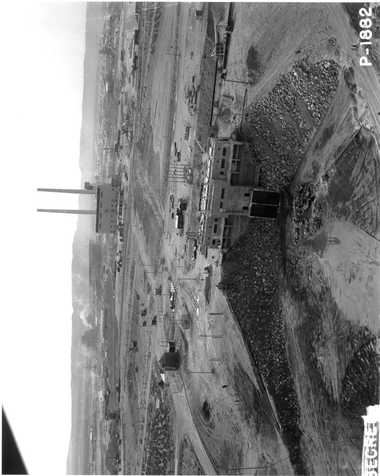
Photograph 12: The 181-B River Pump House under construction in March 1944, with the 184-B Power Plant in the background. View is to the southeast. [P-1882]
