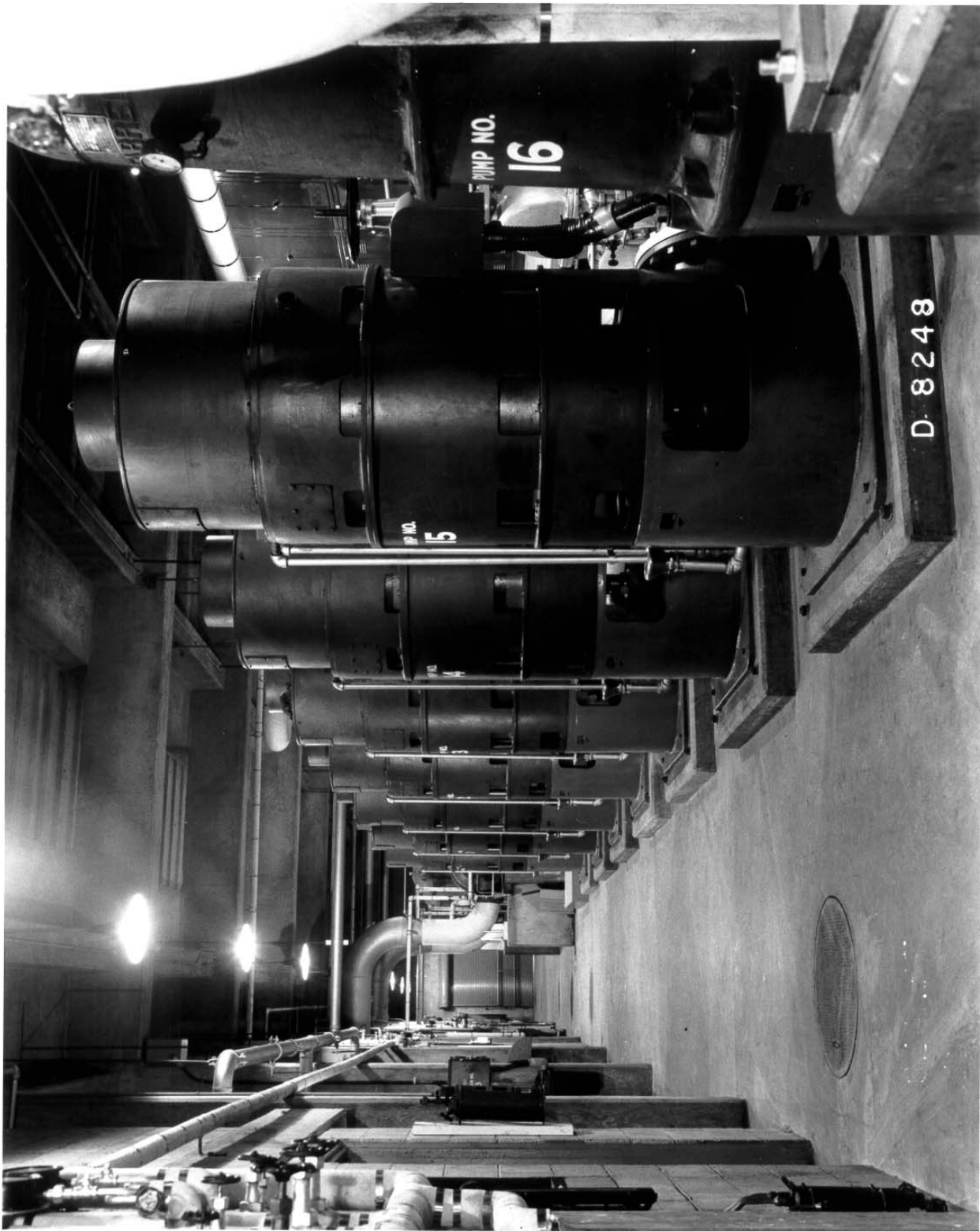
Photograph 13: The River Pump House pump room, in this case in the 100-F Area in January 1945. In the 100 Area, the pumps supplied water to the 100 Area and to the export water system that ran to D and F reactors and the 200 areas. [D-8248]
