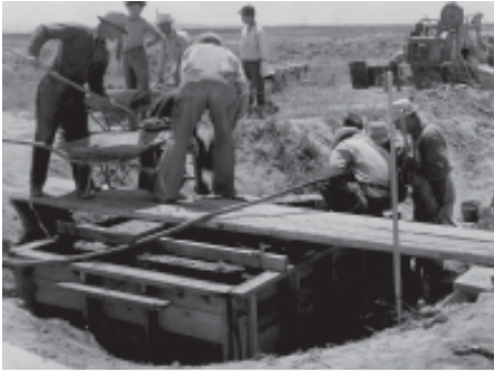
Constructing the irrigation canal controls in Minidoka's agricultural areas. June 27, 1944. National Archives.
