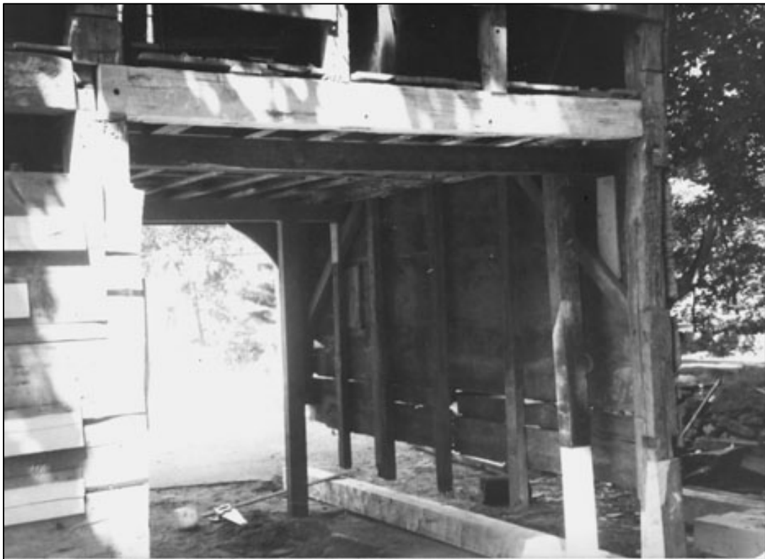
Figure 35. Elisha Jones Shed: East and north wall repairs, including replacement of east- wall girt and north- wall sill, and splicing of posts and studs, 1974.
