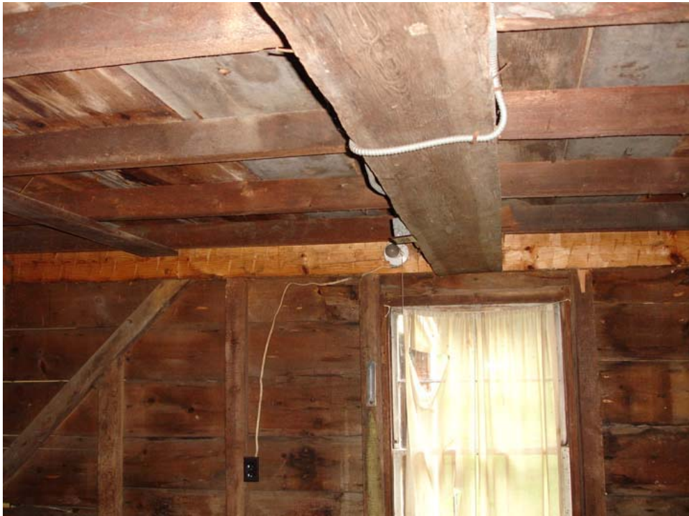
Figure 62. Elisha Jones Shed: Shed Room 104, east wall, exposed framing including summer beam, 1974 replacement girt, studding, and bracing (2006).
