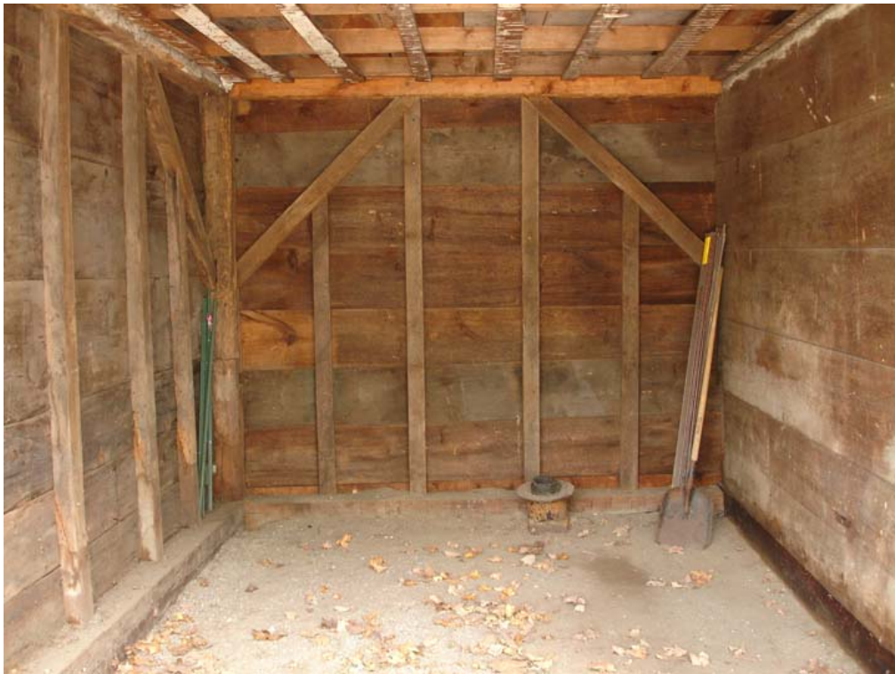
Figure 63. Elisha Jones Shed: Chaise stall, north and east walls, exposed framing including 1974 replacement sill and east girt, spliced studding and corner post, and bracing (2006).
