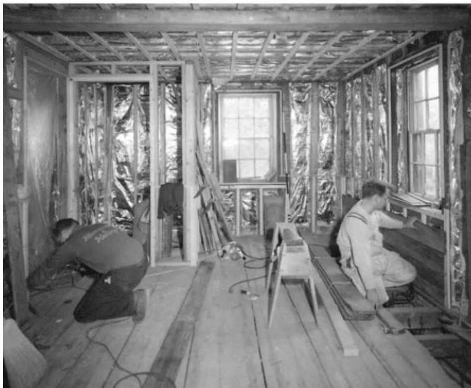
Figure 33. Elisha Jones House: East extension of north lean- to, installation of chestnut wainscoting in kitchen ell during 1966 rehabilitation work.
