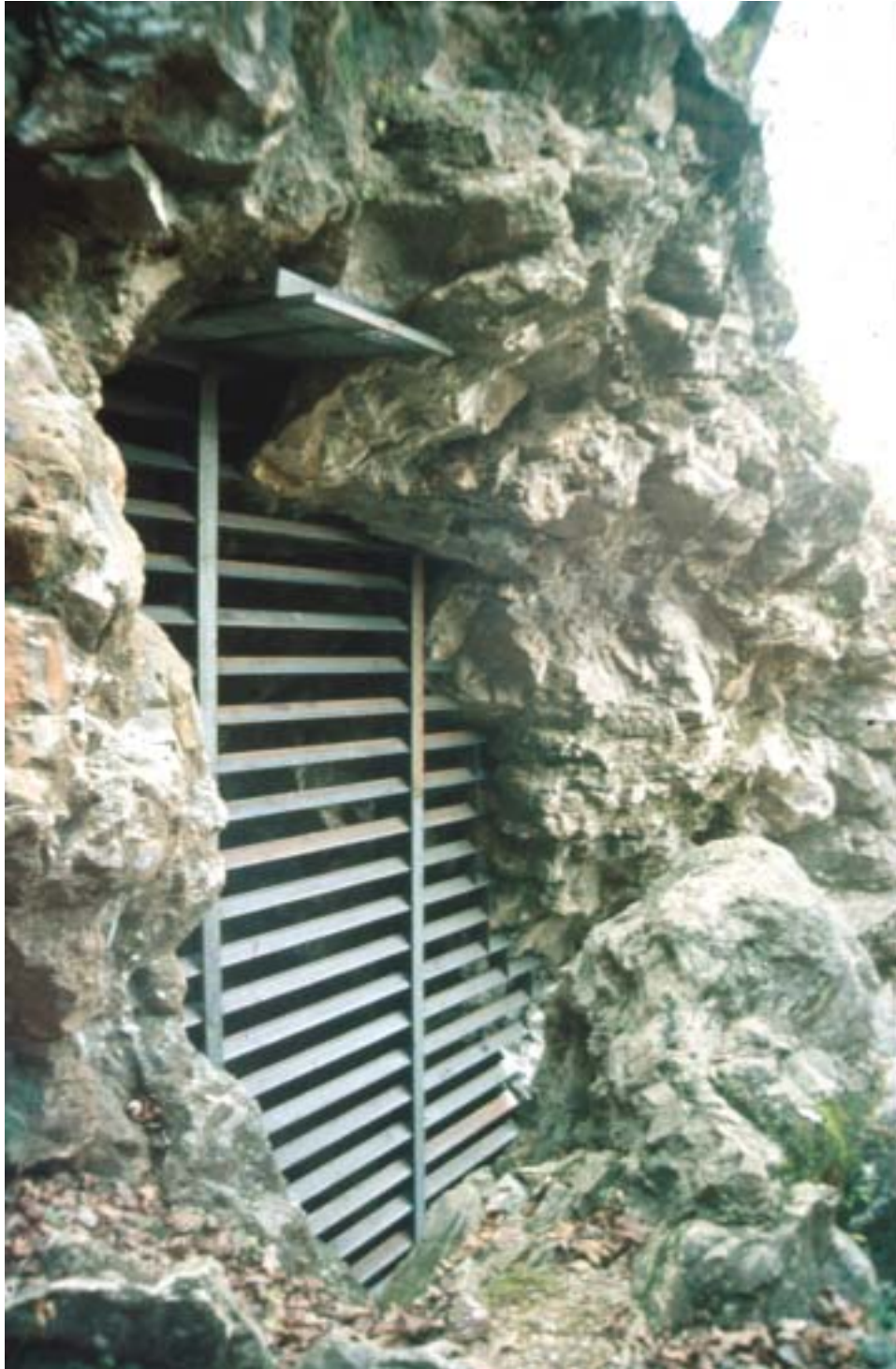
Figure 2. Bat gate installed at Monte Cristo Zinc Mine, Buffalo National River, Arkansas. (1993)
