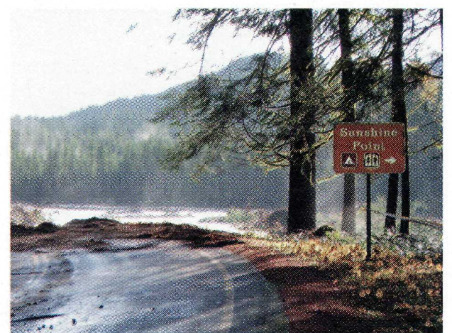
The Nisqually Road was washed out along with the former Sunshine Point Campground
