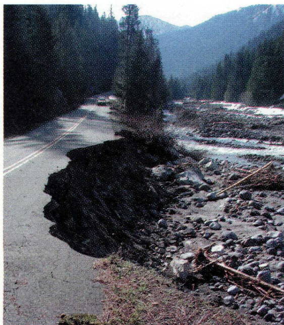
One lane of the road to White River Campground was washed down river.
