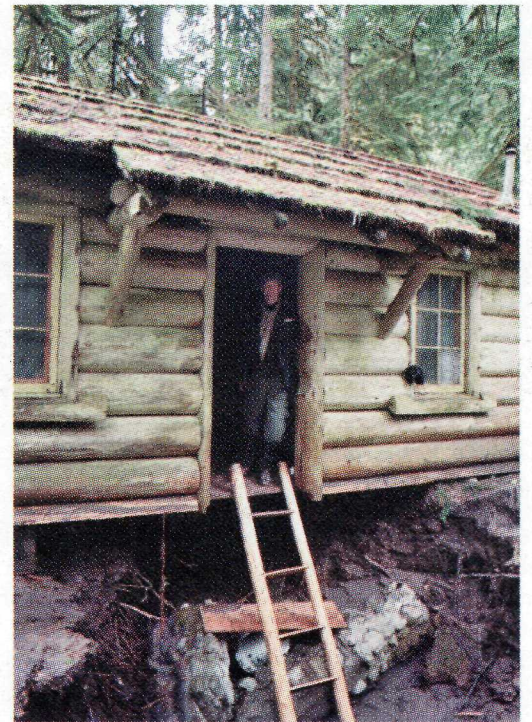
A channel of the Carbon River carried away the ground beneath the historic Ipsut Creek Cabin.
