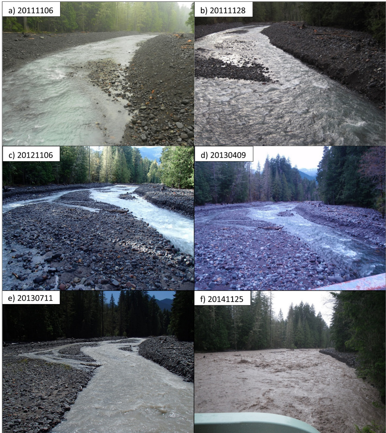
Figure 7. Evolution of the modified channel over three years. Panels (a) through (f) are looking downstream from the bridge deck. The stream flow in (a) through (d) is representative of low-flow conditions. Flow in panel (e) is typical of summer runoff. Panel (f) is near bankfull runoff during a precipitation induced flood (Photos: NPS and US Federal Highways Administration).
