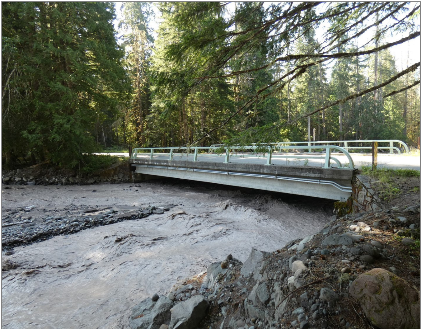
The north side of the Tahoma Creek Bridge, facing south on August 6th, 2019, during a period of increased water stage and sediment transport from an upstream debris flow.
