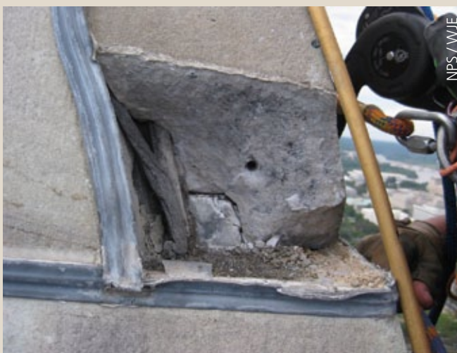
Most of the earthquake damage, like this spall, occurred in the upper 100 feet of the monument.
