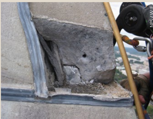
Most of the earthquake damage, like this spall, occurred in the upper 100 feet of the monument.
