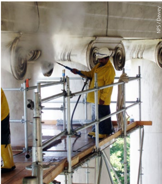
Washing the Thomas Jefferson Memorial to prevent damage from indirect effects of acid rain.
