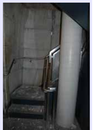
Debris covers the stairs on the museum level.
