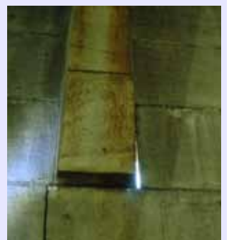
Daylight shines through a crack in the outer wall.
