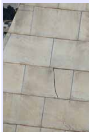
A huge exterior block cracked on the west face.
