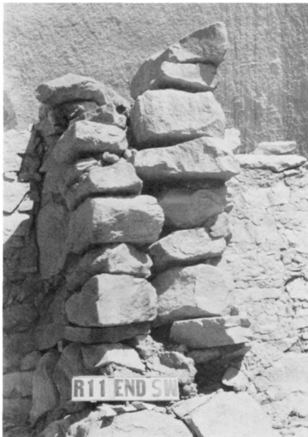
Figure 44. Room 11, job 6, before stabilization, August, 1977.
