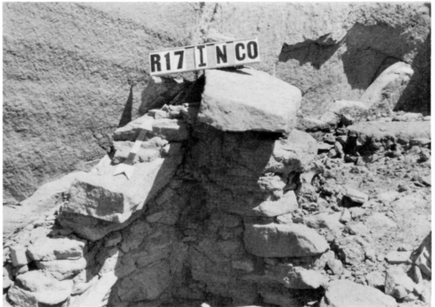
Figure 38. Room 17, job 4, before stabilization, August, 1977.
