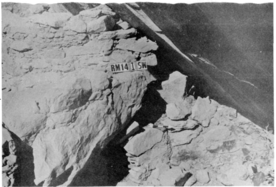
Figure 65. Room 14, job 15 before stabilization, August, 1977.
