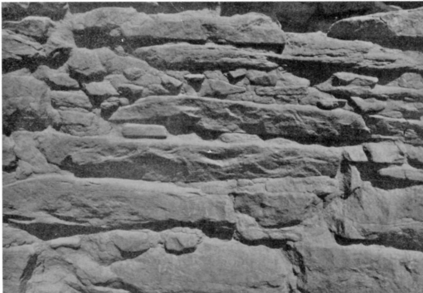
Figure 95. SHP-78 4-4-6. Winter check Room 3, southeast exterior wall. Close-up of painted and methyl methacrylate areas. March 1979.
