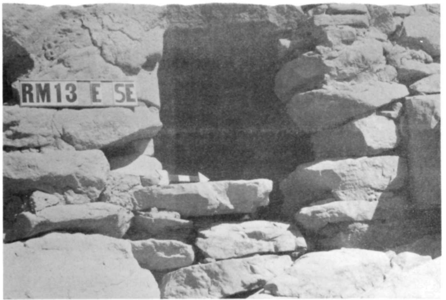
Figure 62. Room 13, job 14 before stabilization, August, 1977.
