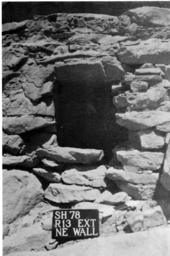
Figure 63. SHP-78 1-10-12. Room 13, job 14 northeast exterior wall before stabilization, May, 1978.
