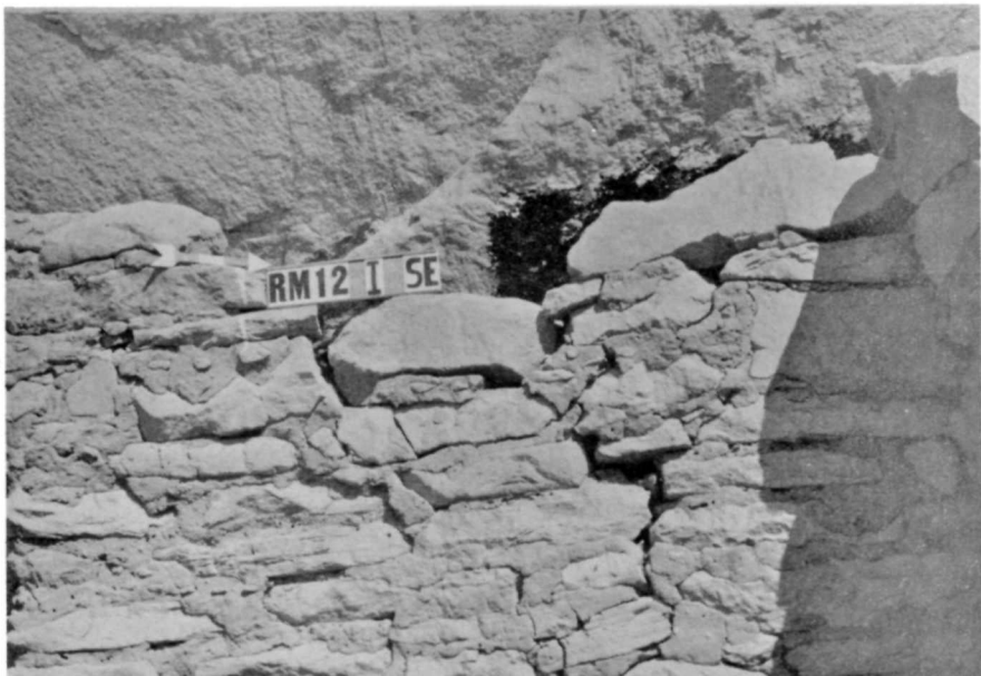
Figure 56. Room 12, job 12 before stabilization, August, 1977.
