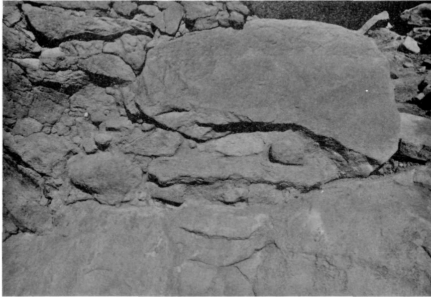
Figure 101. SHP-78 4-8-10. Winter check. Room 14, job 16, northeast exterior wall; close- up of soil mortar. March 1979.
