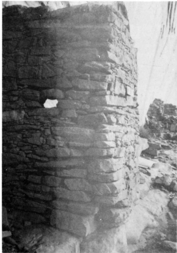
Figure 28. Room 3, job 1 before stabilization, August, 1977.
