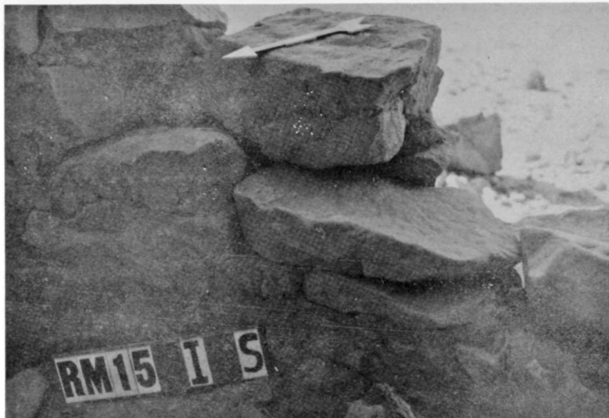
Figure 76. Room 15, job 19 before stabilization, August, 1977.
