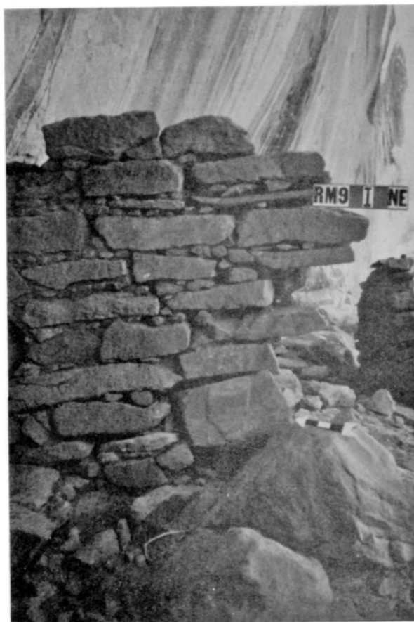
Figure 41. Room 19, job 5, before stabilization, August, 1977.
