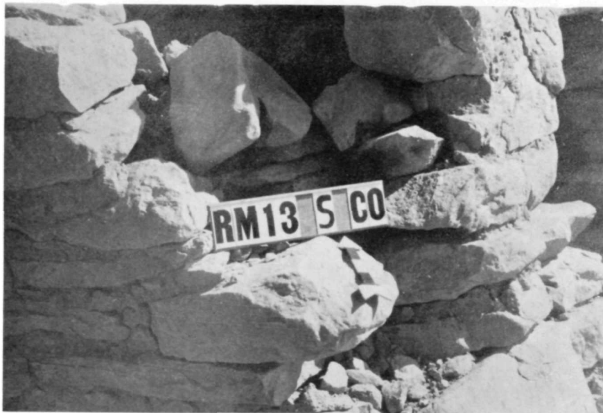
Figure 59. Room 12, job 13 before stabilization, August 1977.
