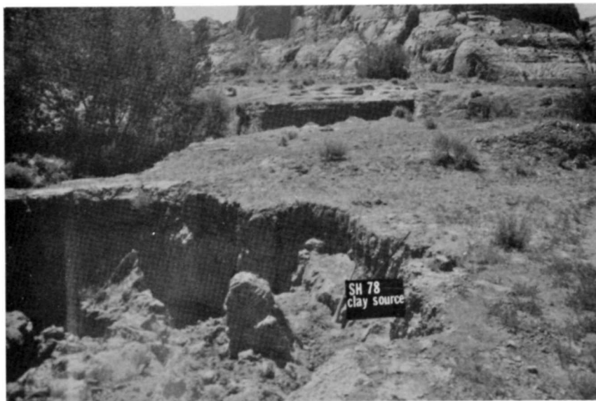
Figure 8. Same sinkhole with mine, but different vein- used for the last part of stabil- ization.
