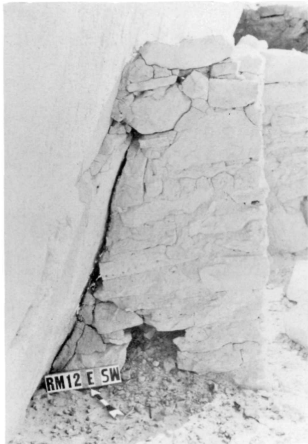
Figure 53. Room 12, job 10-11 before stabilization, August, 1977.
