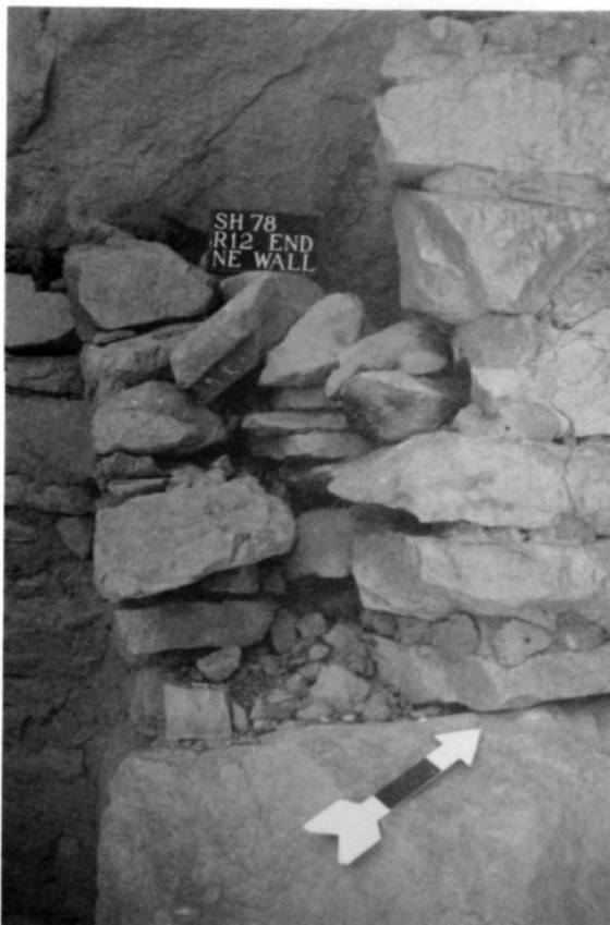
Figure 60. SHP-78 1-21-23. Room 12, job 13 northeast end wall before stabilization. May, 1978.
