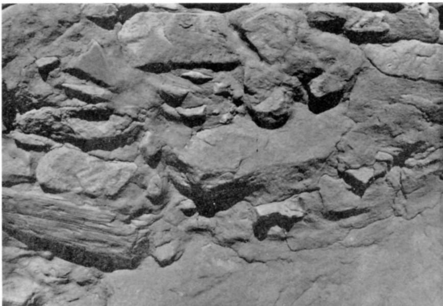
Figure 97. SHP-78 4-7-9. Winter check Room 3, southeast interior wall. Close-up of beam seat area. March 1979.
