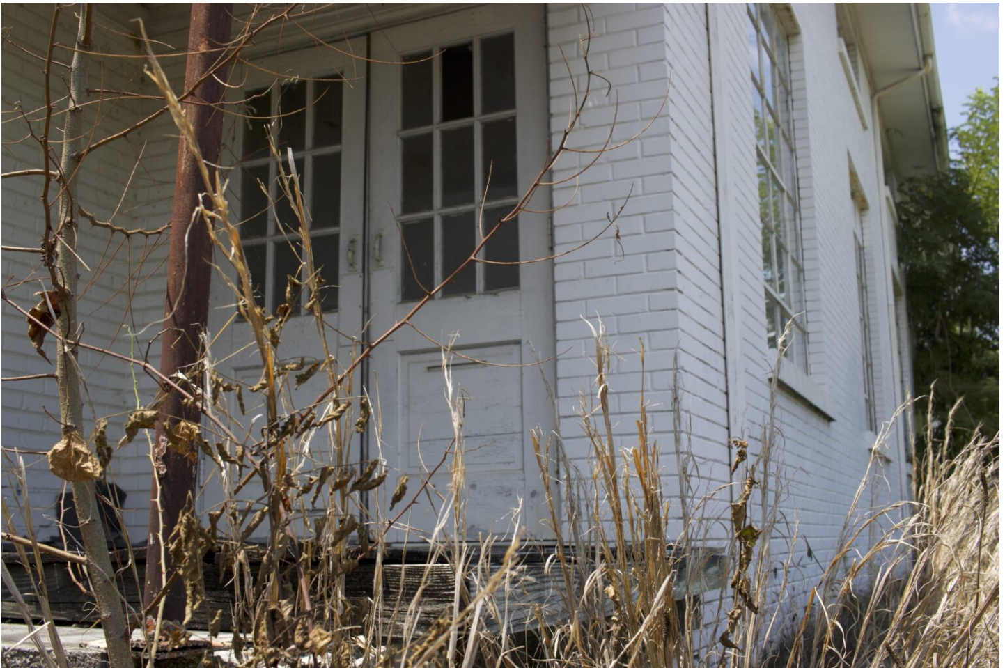
📷 Empty since 1964, the West Gaines School building is in need of a new roof, new gutters and removal of overgrown grass and bushes. (Photo: Lonnie Lee Hood)
