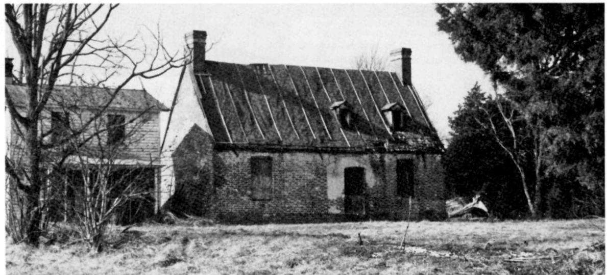
Resurrection Manor, St. Mary's County, Maryland. This early 18th century brick house is located on one of the earliest manorial grants made in Maryland. Vacant for years, its structural and material integrity threatened, Resurrection Manor may succumb to demolition if the remaining seven acres of land are sold for waterfront housing and no new owner can be found who is willing to preserve the manor house. Photo by Jean E. Travers.
