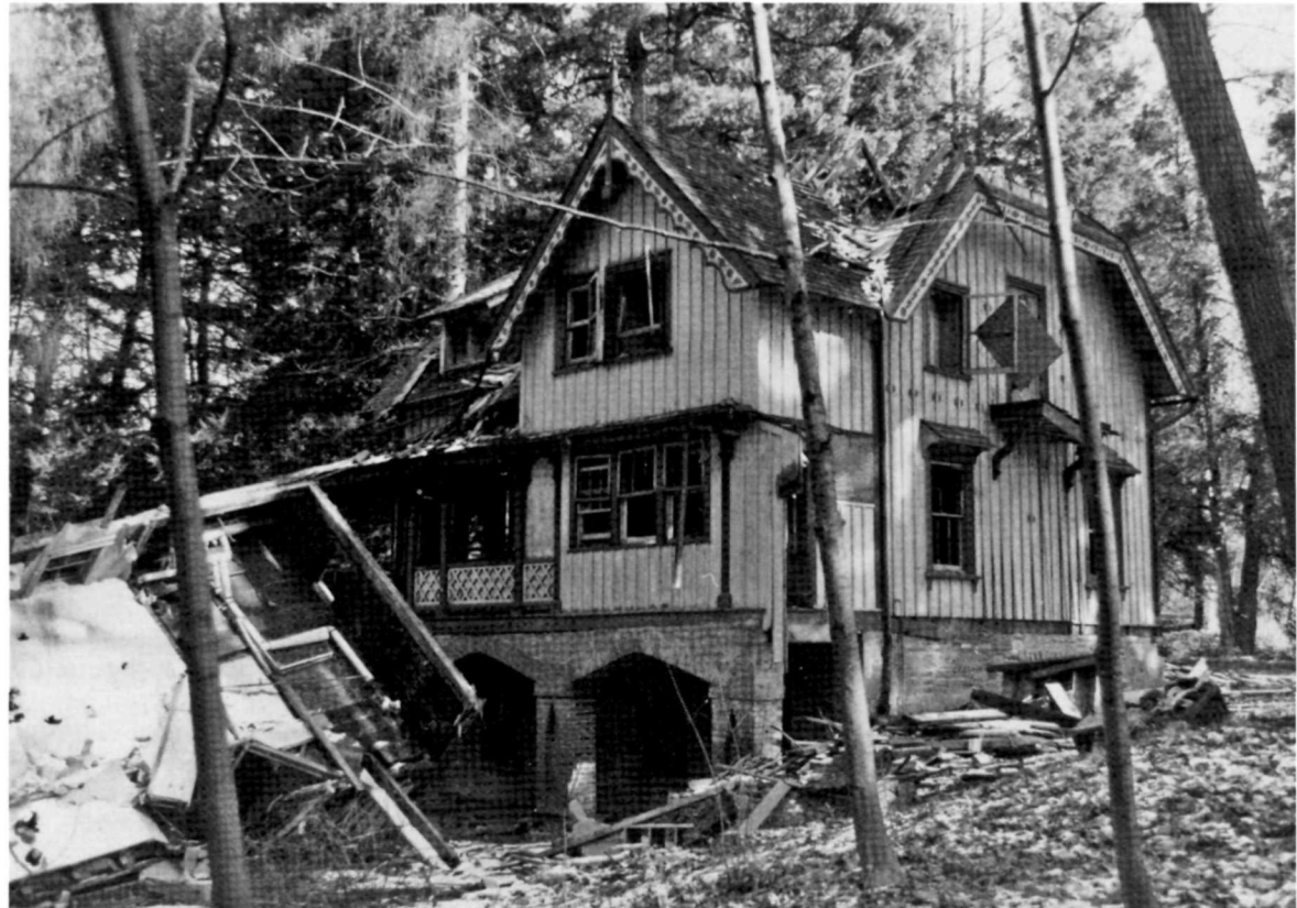
Matthew Vassar Estate, Poughkeepsie, New York. This property was designed for the founder of Vassar College by Andrew Jackson Downing, foremost American landscape architect in the mid 19th century. The former owner of this property at the time of its Landmark designation demolished several of the historic structures on the estate. Photo by James Dillon.
