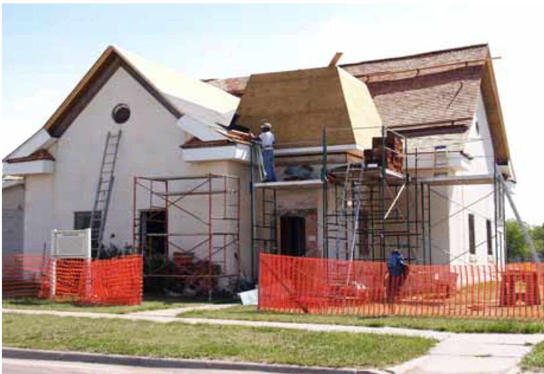
Figure 16. First Baptist Church during stabilization, 2006. Nicodemus NHS Collection, Acc no. 22, Catalog no. 20.
