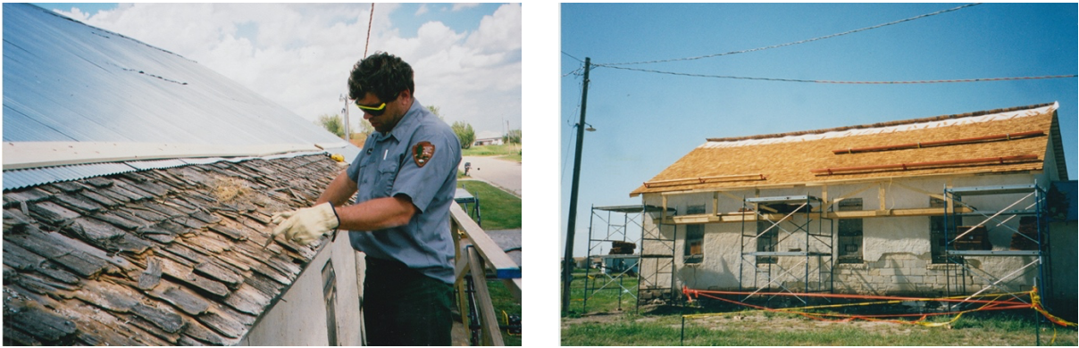
Figure 12. Repairing the roof on the AME Church, 2001. Nicodemus NHS Collection, Acc no. 22, Catalog no. 20.
