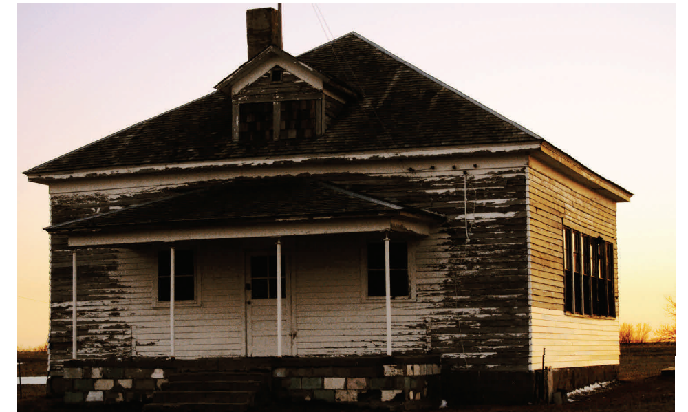
Once easements are signed, restoration work on the District #1 Schoolhouse can begin. (William Pope, NPS)
