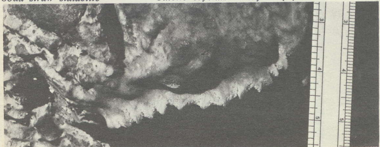
Stalactites formed since exit tunnel was completed in 1933
