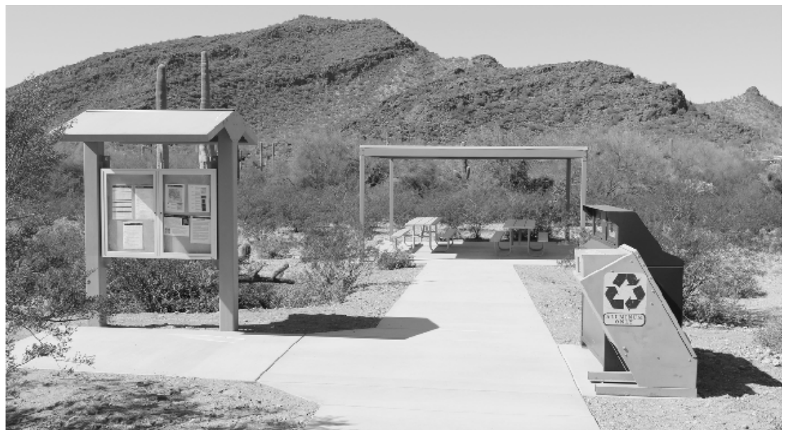
Newly constructed ADA accessible picnic area at the Kris Eggle visitor Center.
