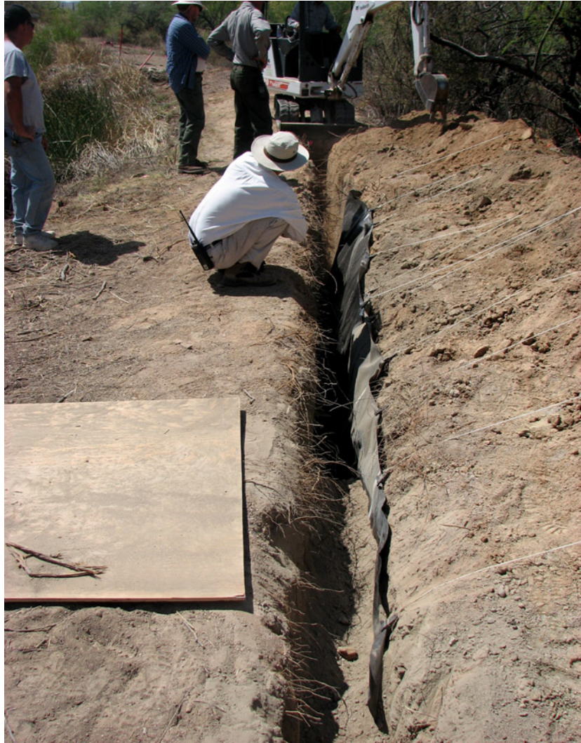
Figure 14. Progression of diaphragm wall construction. Trench in background is being excavated, in the middle ground is ready for backfilling, and in foreground has been backfilled with dry concrete. April 30, 2008. Organ Pipe Cactus National Monument, Arizona.
