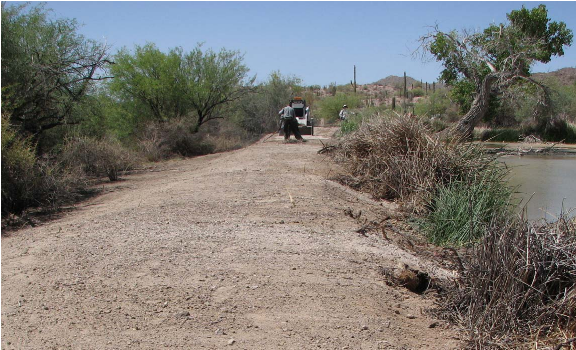
Figure 6b. The retaining berm after clearing trees and shrubs and installing the diaphragm wall. View is from approximately the same point as Figure 6a. Note leaning cottonwood tree in upper right. May 1, 2008 Quitobaquito Pond, Organ Pipe Cactus National Monument, Arizona.
