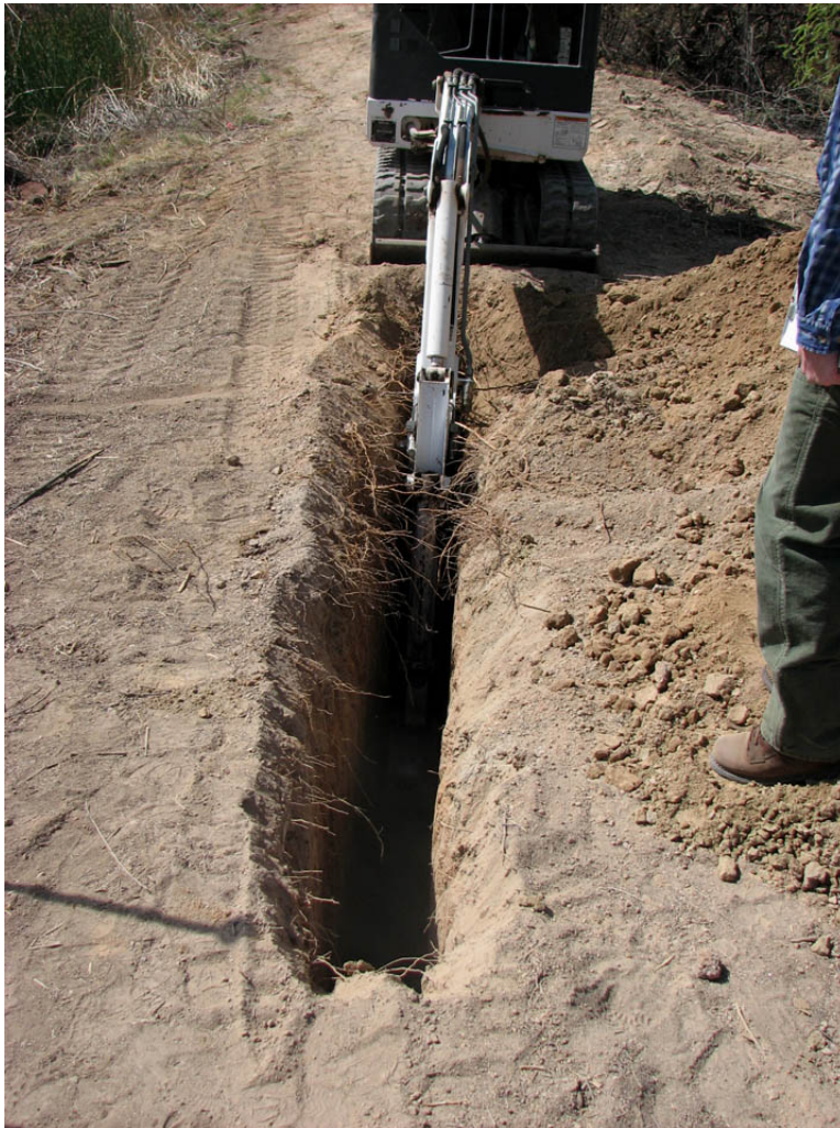
Figure 10. Excavating trench for installing a diaphragm wall in the retaining berm. April 29, 2008. Quitobaquito Pond, Organ Pipe Cactus National Monument, Arizona.
