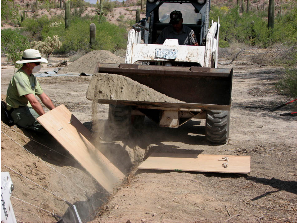
Figure 13. Pouring dry concrete mix into diaphragm wall trench. April 29, 2008. Retaining berm, Quitobaquito Pond, Organ Pipe Cactus National Monument, Arizona.
