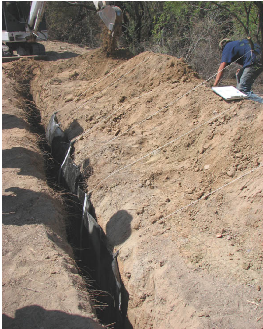
Figure 12. Pond liner material is suspended against the outer wall of the trench, to form a supplemental water barrier. April 30, 2008. Quitobaquito Pond, Organ Pipe Cactus National Monument, Arizona.
