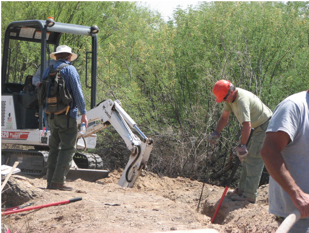
Figure 11. Worker on the right is using pole pruner to trim roots in the trench for diaphragm wall in the retaining berm. Worker standing on the left is an archaeologist monitor examining excavated earth for cultural resources. April 29, 2008. Quitobaquito Pond, Organ Pipe Cactus National Monument, Arizona.
