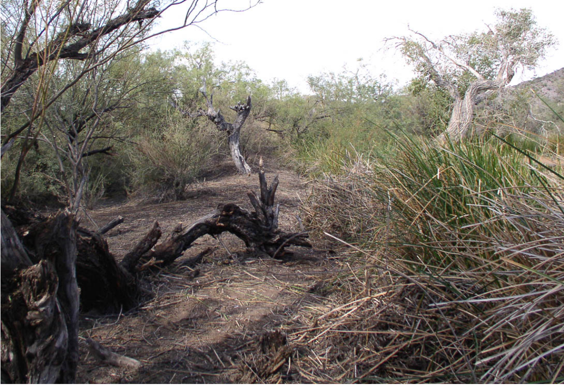
Figure 6a. The retaining berm, view to the northwest from near the spillway. Note the leaning cottonwood in upper right. Understory shrubs and dead lower tree branches had been removed to allow this view. Note large mesquite trees rooted in the berm. November 15, 2007. Quitobaquito Pond, Organ Pipe Cactus National Monument, Arizona.
