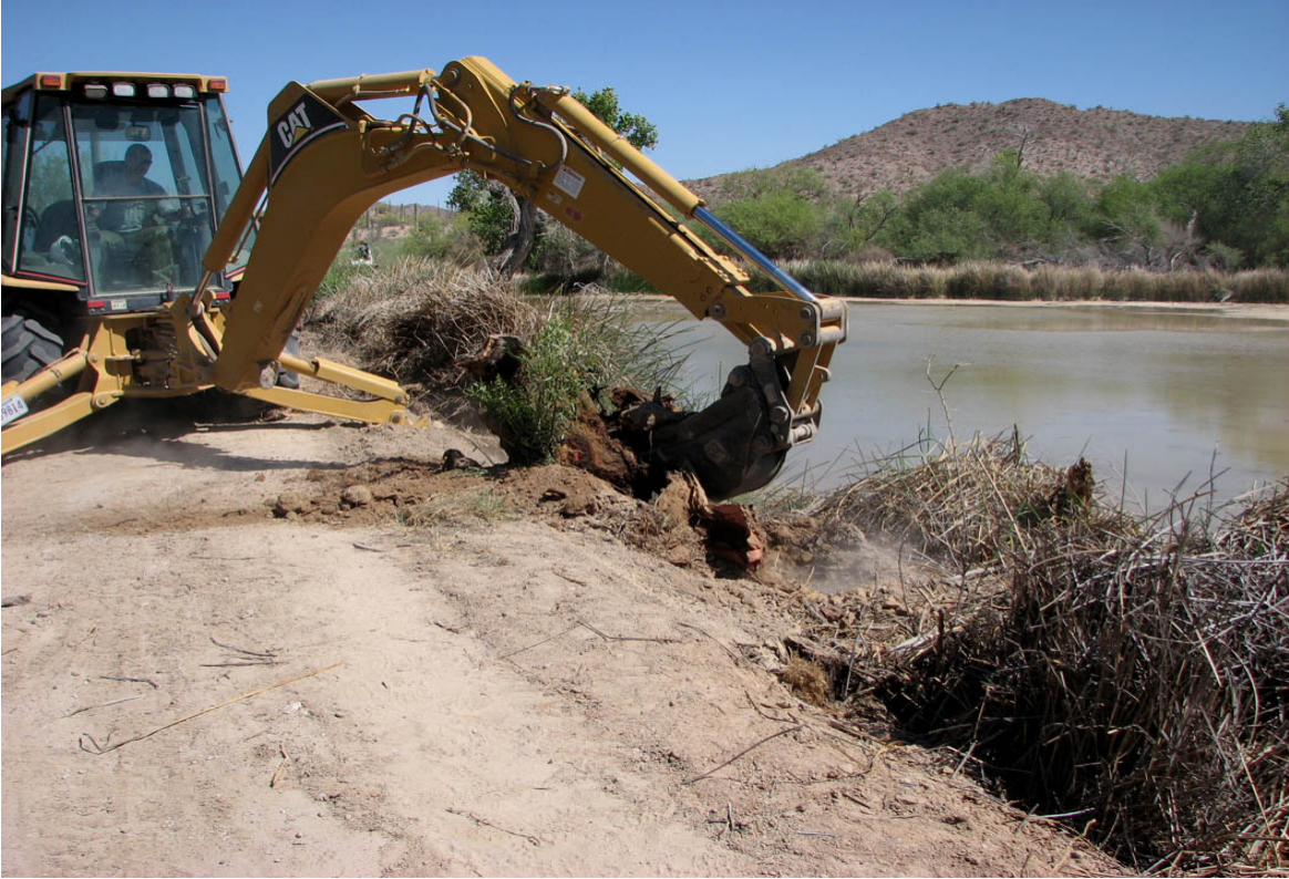
Figure 7. Removing “bee willow” stump and roots from the inner side of the retaining berm. May 5, 2008. Quitobaquito Pond, Organ Pipe Cactus National Monument, Arizona.
