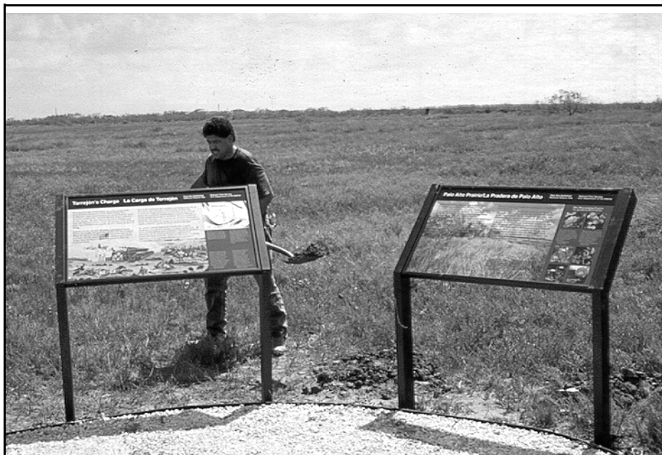
Park volunteer Jesse Camarillo completes the installation of wayside exhibits at the end of the park's interpretive trail. The displays provide information about the prairie and battle activities that occurred near this overlook.
