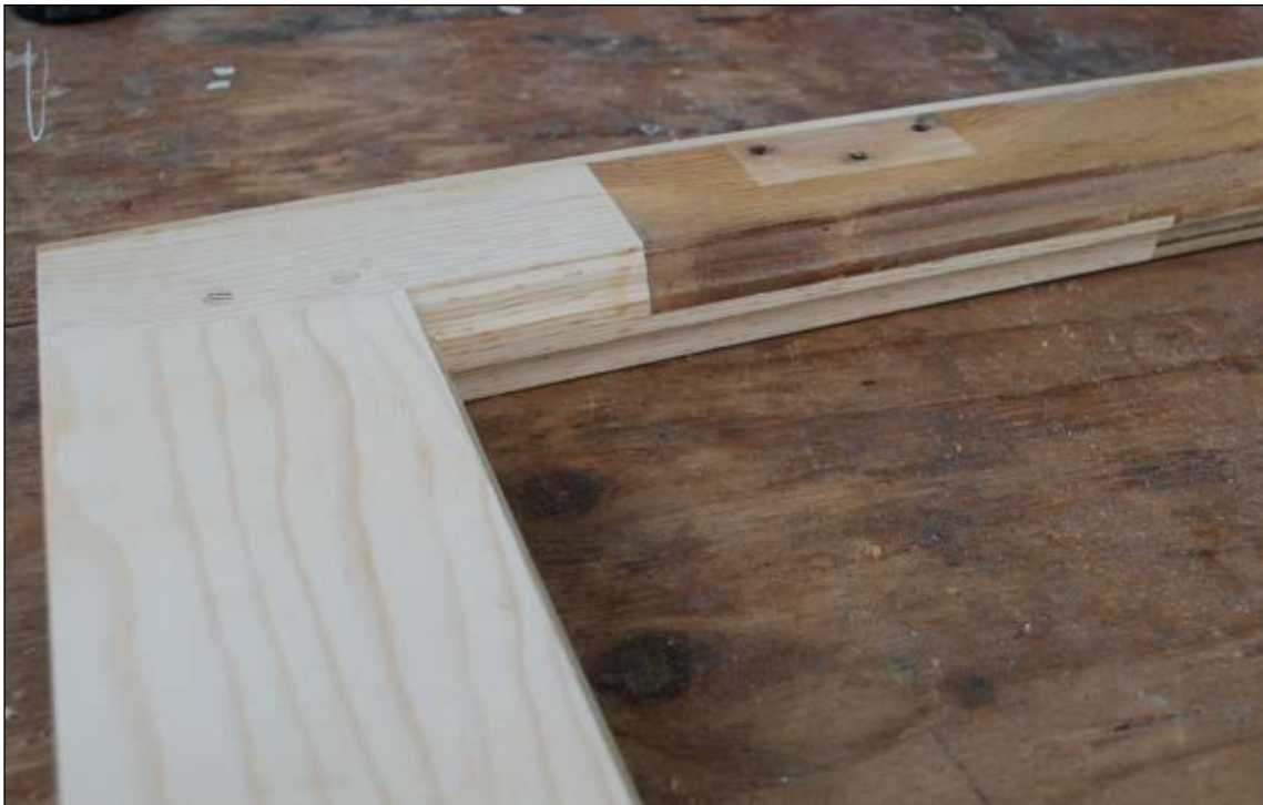
Figure 7. Corner of repaired casement window sash showing lamination, stile extension, replacement of a rail, and wooden dowels to secure the mortise and tenon joinery.
