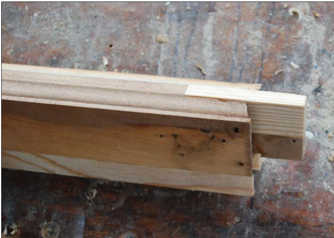
Figure 3. Repaired rail with lamination along full length of outside edge and partial replacement of tenon.
