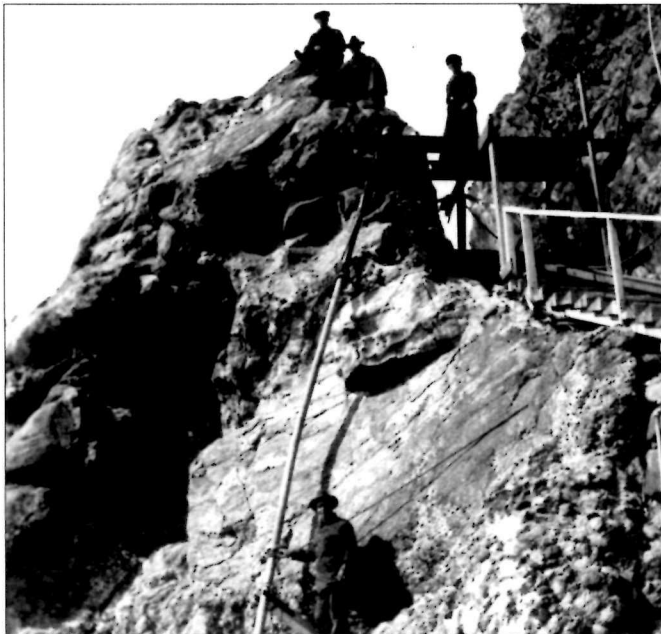
Building the stairs down to the original foghorn building, another 150 feet below the lighthouse level.
