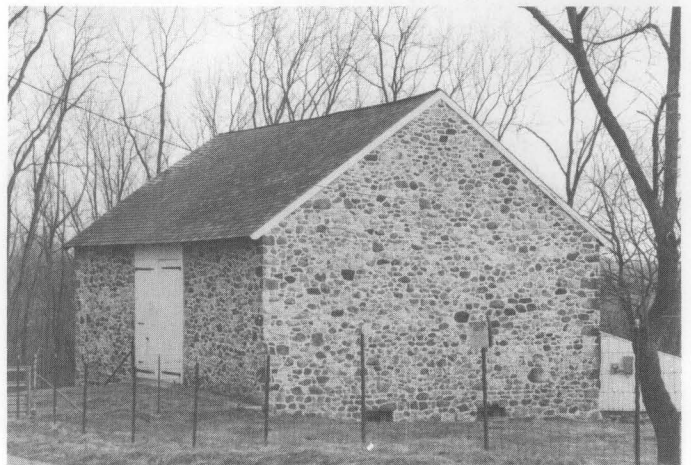
Fig. 3. The stone walls of this Delaware barn are its most notable feature. Built about 1810, the barn is a bank barn. Photo: Valerie Cesna, Delaware Bureau of Archeology and Historic Preservation.
