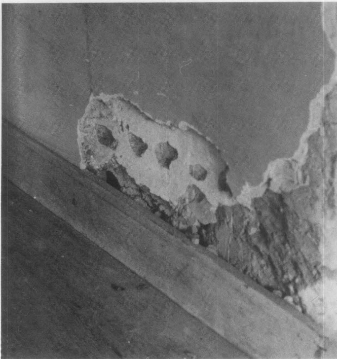
Fig. 4. The builders of this mid-18th century house installed the baseboard moulding first, then applied a mud and horse hair plaster (called paling ) to the masonry wall. Lime was used for the finish plaster. Also shown are the hacking marks which prepared the wall for a subsequent layer of plaster. Photo: Kay Weeks.
