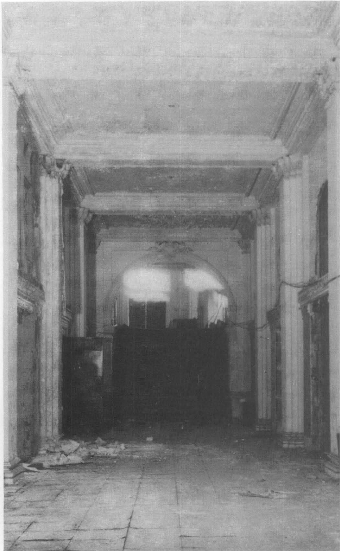
Fig. 13. Water intrusion and freeze/thaw cycles caused extensive efflorescence and ornamental plaster failure. The plaster needed almost total replacement within the rehabilitation project. Photo: Commercial Photographics.
