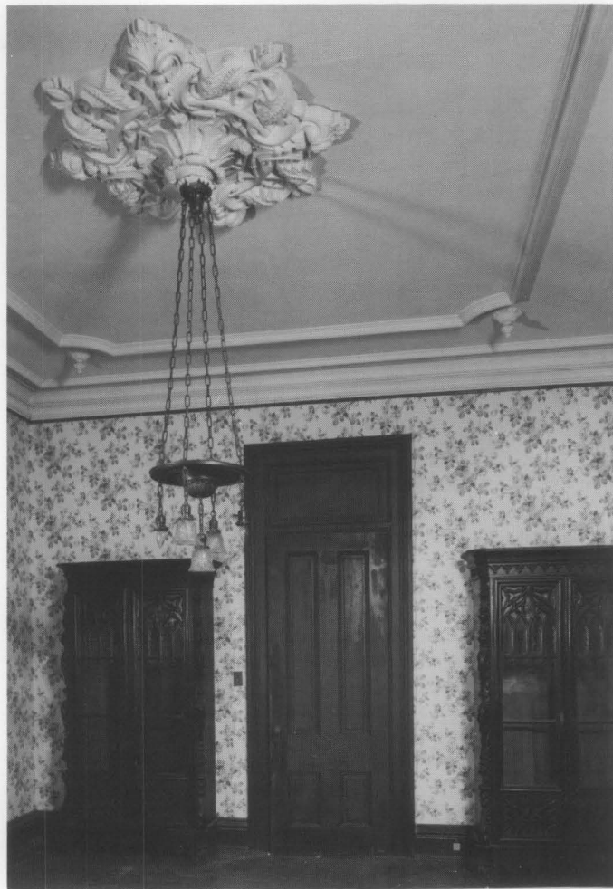
Fig. 2. This parlor medallion and pendant drops shown in a mid-19th century row house in Annapolis, Maryland were originally ordered from a catalog. A local plasterer ran the plain cornice and band ribbon, the curved corners of which were bench run, set with a plaster adhesive and pointed at the joints. Photo: M. E. Warren.
