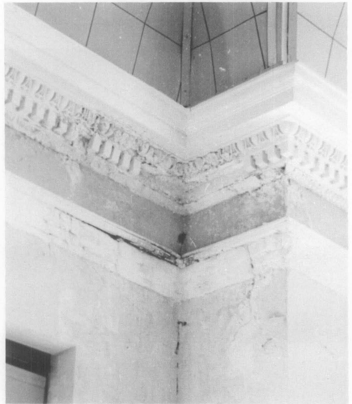
Fig. 11. The cornice of an Iowa courthouse has been severely damaged from a roof leak. In order to repair the ornamental plaster, a thixotropic rubber impression will be taken (with the paint build-up undisturbed). The efflorescence will be removed and fresh plaster casts installed so that egg and dart, dentil and leaf molding are perfectly aligned. Photo: National Park Service files.
