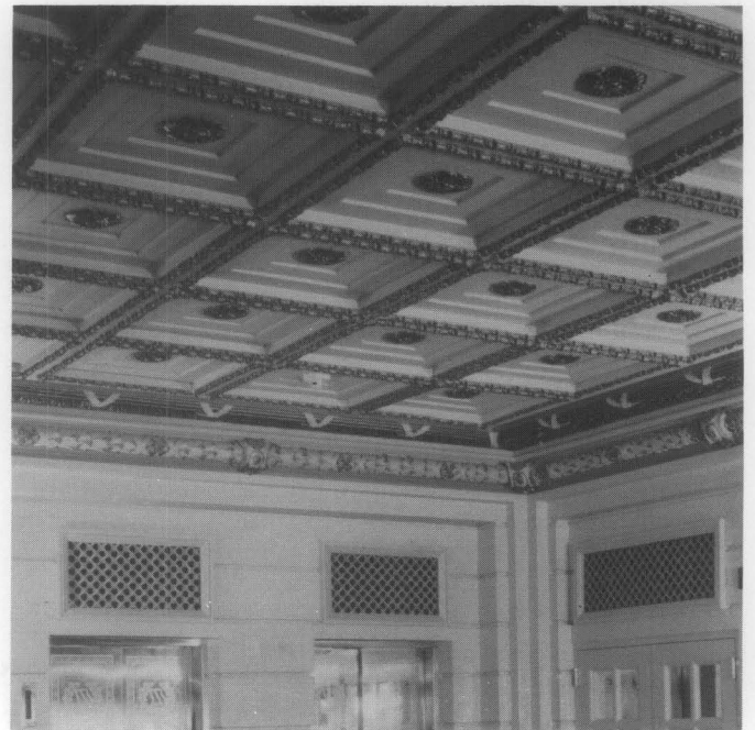
Fig. 9. The elaborate coffered ceiling was designed for the Willard Hotel in Washington, D.C. (1902-04) by Henry Janeway Hardenbergh. The coffered ceiling was restored as part of a rehabilitation project in the 1980s. Photo: Carol M. Highsmith.
