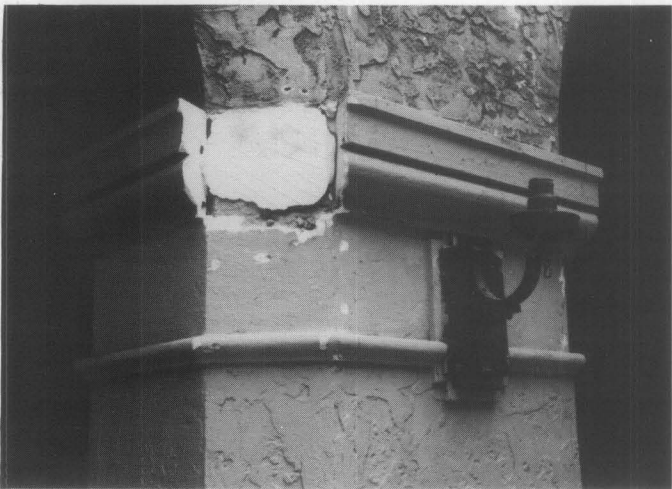
Fig. 14. A mitered portion of this impost capital abacus has fallen, revealing the plaster adhesive material. Repairs are made by obtaining a section through the abacus, making a bench-run length, cutting, fitting, and readhering the missing piece. Finally, the joints are pointed. Photo: Lee H. Nelson, FAIA.
