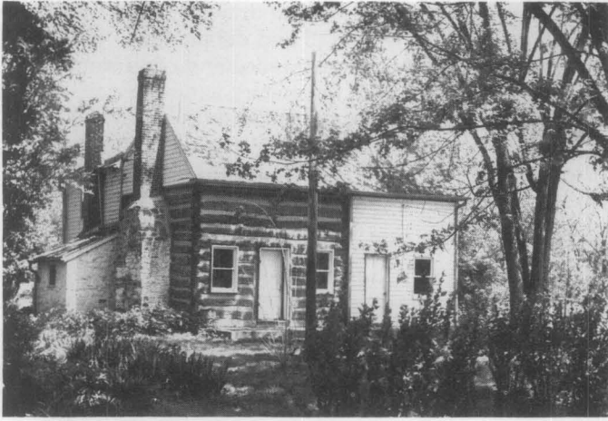
Fig. 13. Historic wood clapboard siding originally applied to conceal the fact that this house was built in two sections of different materials has been inappropriately removed from the 1793 log portion. Photo: National Park Service Files.
