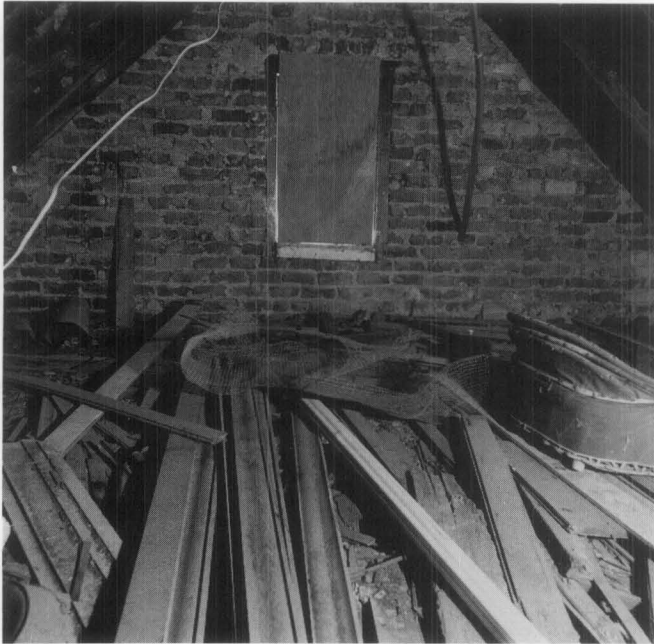
Figure E. Discarded items are routinely stored within attics, then forgotten, only to be discovered during a later investigation. Seemingly worthless clutter and debris may help answer many questions. A thorough inventory should be performed before evaluating any object's usefulness.
