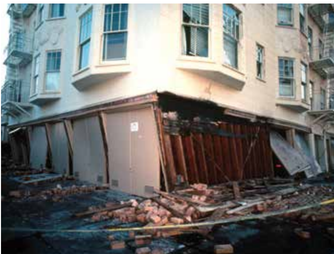
Figure 30. Large perimeter openings and a limited number of interior partitions on the ground floor can create a “weak story” condition that makes buildings particularly vulnerable to earthquake damage. Photo: USGS.
