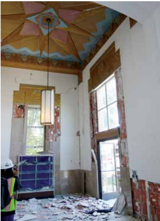
Figure 6. Failing nonstructural elements such as the stone-veneer window and door surrounds shown in this image can become a life-safety hazard when they block or impede an exit path. Photo: Wiss, Janney, Elstner and Associates, Inc.
