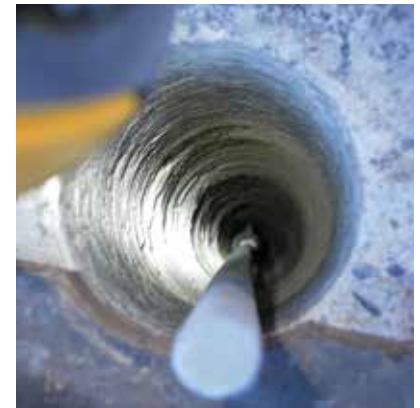
Figure 25. View of one of the center cores drilled down through the wall.
