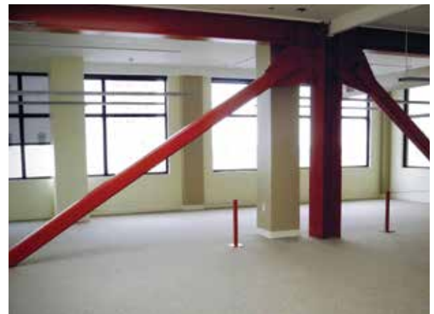
Figures 4-5. Using moment frames (horizontal and vertical steel members identified by the arrows) set back behind storefront openings as seen in Figure 4 (left), or placing brace frames (in red) away from the windows as illustrated in Figure 5 (right) are solutions that meet historic preservation goals. Figure 4. Photo: Elizabeth Hilton.
