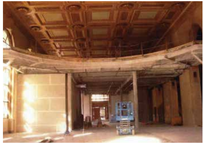
Figure 12. A mezzanine was added to the original banking hall of this 1921 former bank building as a seismic strengthening measure. Subdividing such an important character-defining space can result in a severe loss to a building's historic integrity.
