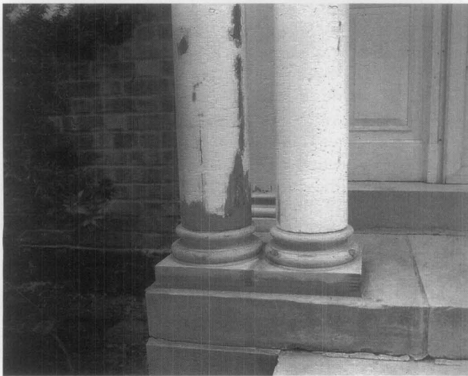
Figure 11. The lower shaft of the porch columns had decayed as water wicked up through the end grain (top). The column shafts were repaired in place by cutting out the deteriorated wood and making repairs using epoxy consolidants and fillers. (bottom). The column bases were replaced. Photos: Paul Marlowe, Marlowe Restorations.
