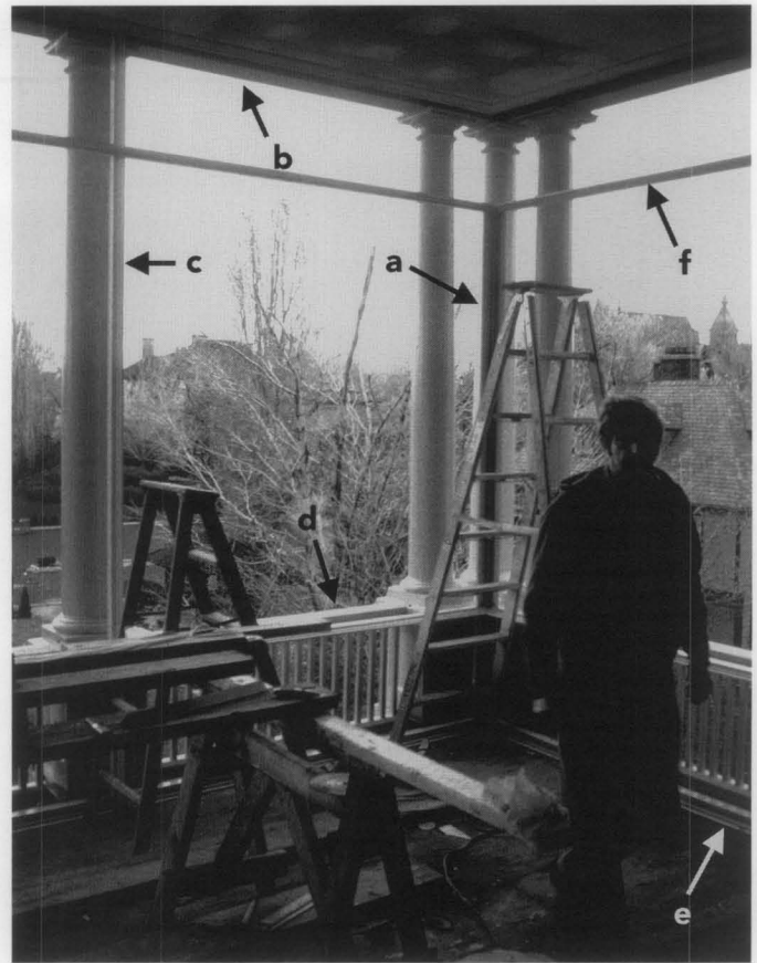
Figure 16. The use of near full glazing to enclose a porch may be appropriate depending upon the historic character of the building, location of the porch, how the interior space is to be treated, and other factors. This enclosure of a rear porch to create a conference room successfully utilizes large expanses of glass and narrow metal framing set behind existing porch elements (a through e). Where an additional horizontal support was needed (f), the frame was placed at a location that is found in many traditional insect screen enclosures. Photo: Charles Fisher.
