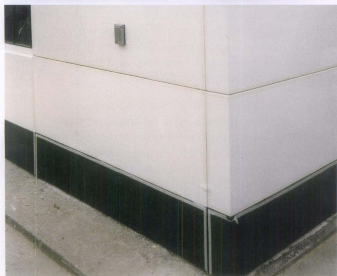
Figure 11. The porcelain enamel facade of this former Texaco station (1960) had numerous dents and scratches that had exposed the steel beneath the enamel to deterioration (top). Rehabilitation work included repairing localized damage to the panels and blending patched areas to match adjacent historic material, replacing sleepers beneath the panels (center), replacing severely damaged panels with like material, and recaulking the joints (bottom). Photos: John Vaughan, Architectural Conservation Services.
