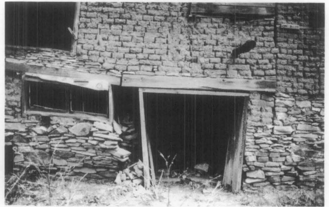
Structural Damage and Cracking. Sagging, bulging, and cracking of walls and roofs are signs of serious problems in the adobe building. It is always advisable to secure professional services in the repair of such problems. (National Park Service)
