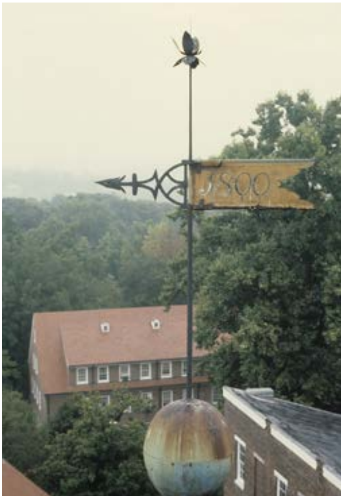
Figure 8. Church steeples, roof turrets, and chimneys were identified early on as being susceptible to lightning strikes. Finials, weathervanes, and other such ornamentation in these locations could often serve as lightning rods when connected to down conductors and grounds. The cupola on the Home Moravian Church in Winston-Salem, North Carolina, is an excellent example. Old Salem, Inc., has a number of Moravian buildings where early lightning protection systems are still in place. Photo: Sunni L. Goodson.
