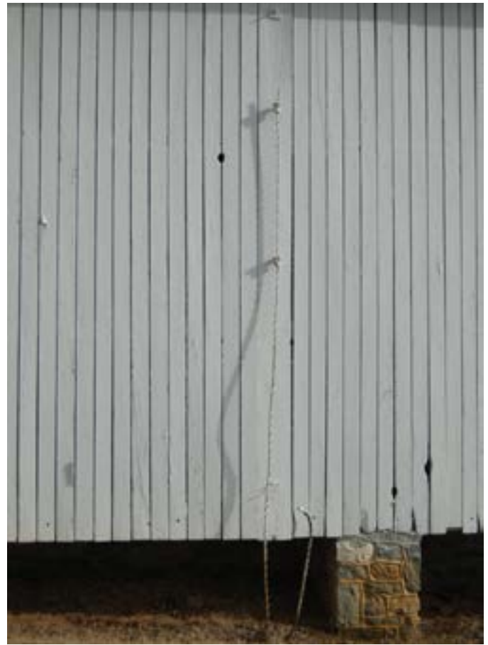
Figure 14. Lightning protection systems should be visually inspected every year and once every five years be inspected by an experienced professional. Note the break in the down conductor at the top of the photograph and the lack of a bonded connection to the cable at the bottom, which goes to one or more grounds. The old ground rod should be bonded to the new ground. Photo by author.
